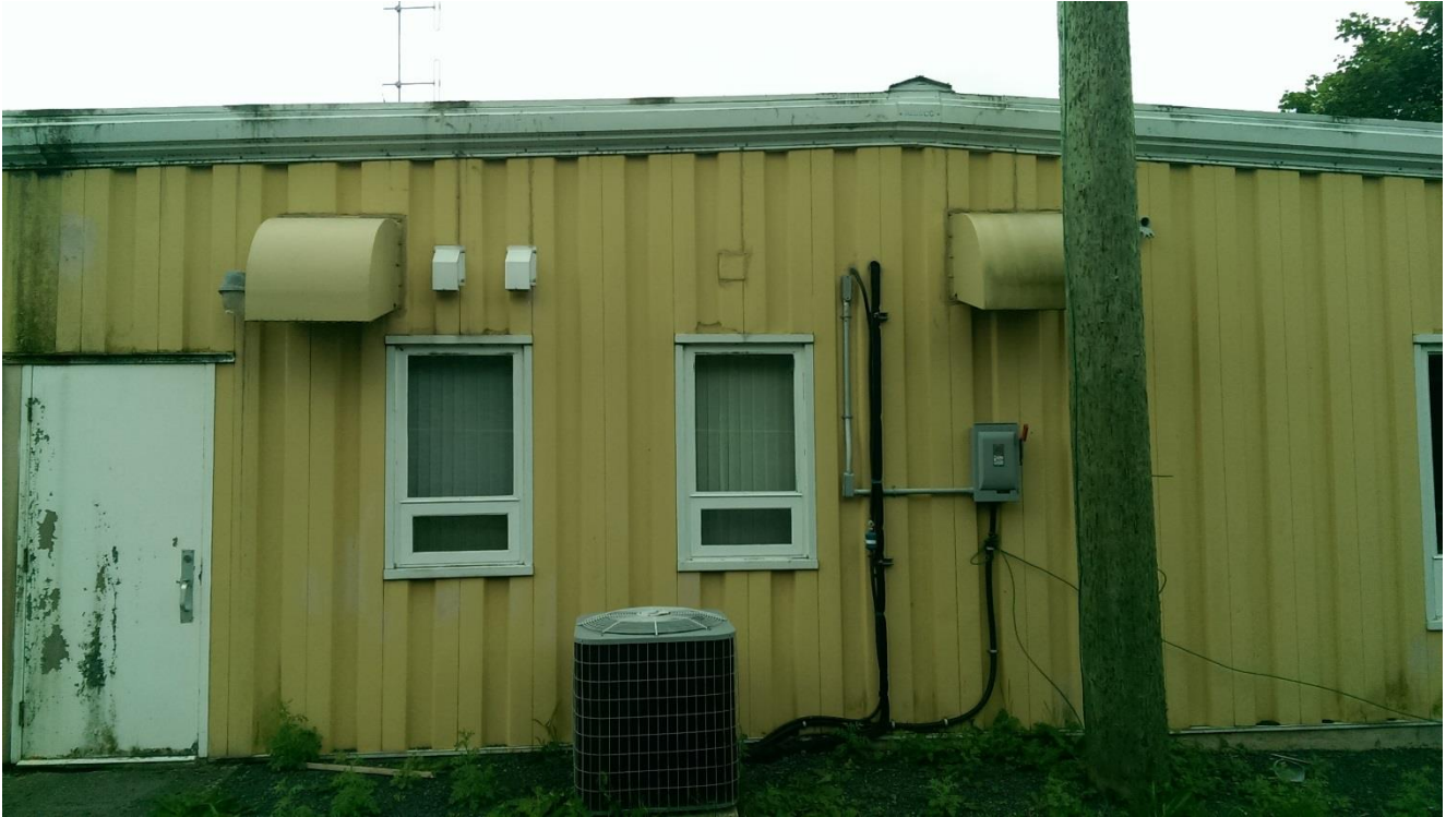
Photo 19 - AC Condenser and Air Intake and Exhaust Hood
