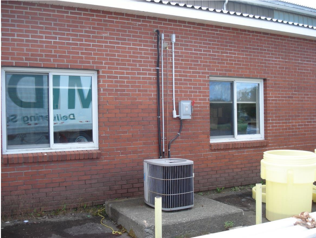
Photo 27 - Front Office Area Condenser Unit
