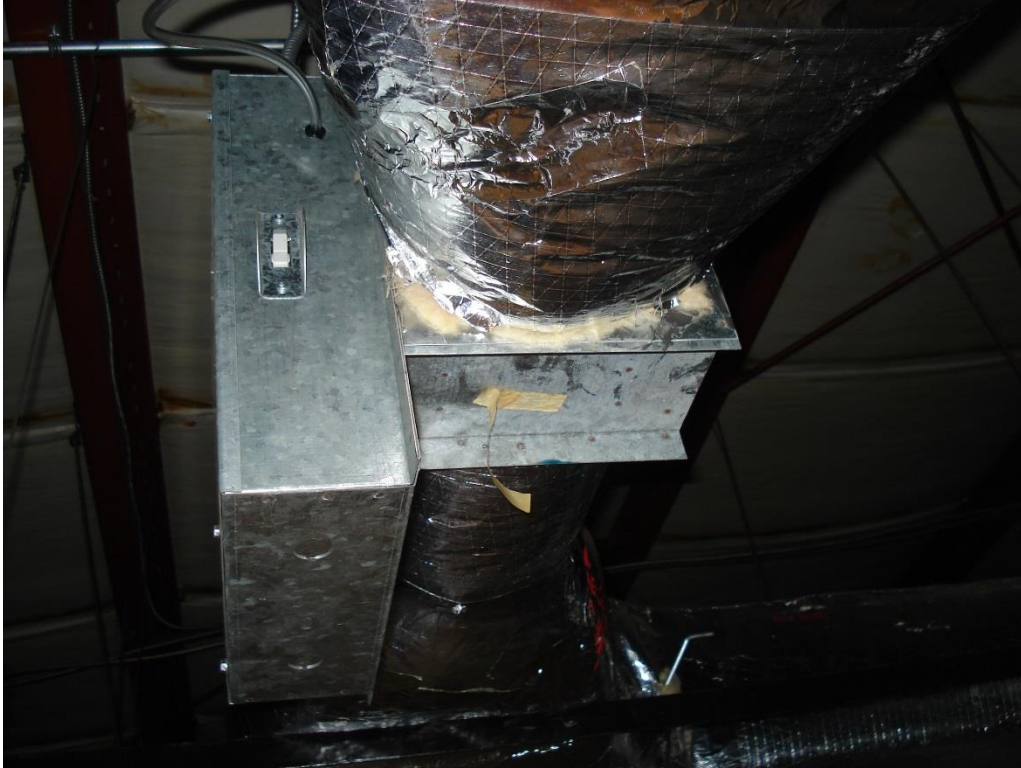
Photo 23 - Zone Duct Heater
