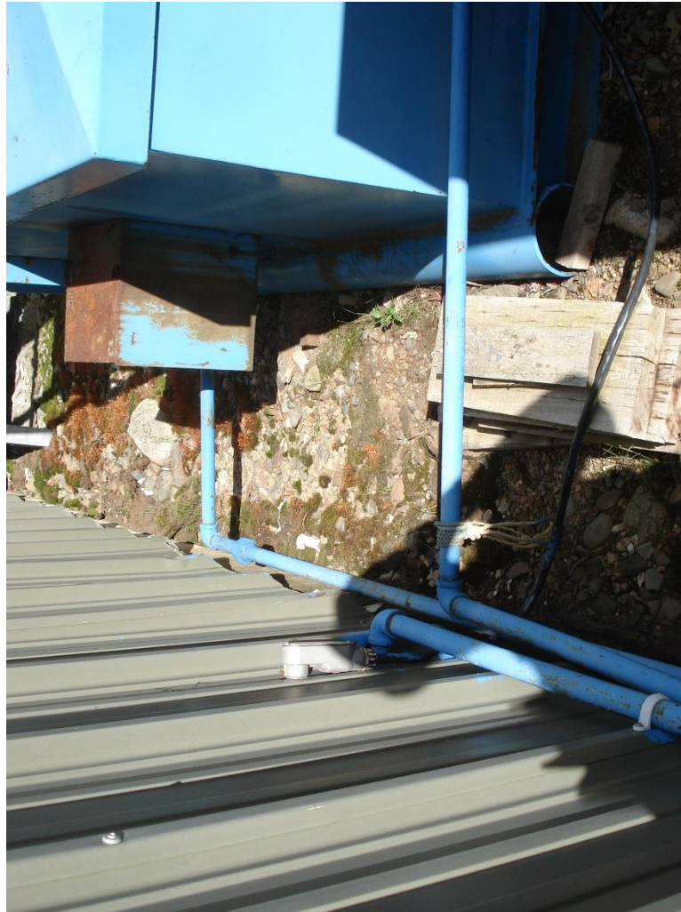
Photo 17 - Tank Piping Not Properly Supported
