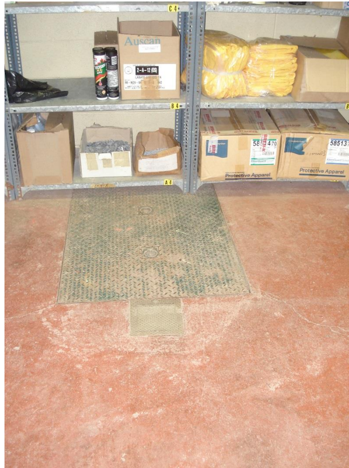
Photo 5 – Oil Interceptor Access Cover
