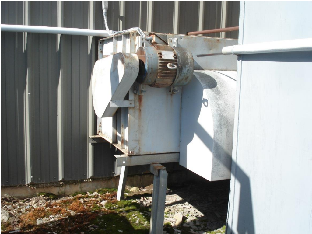
Photo 34 - Paint Room Make-up Air Unit
