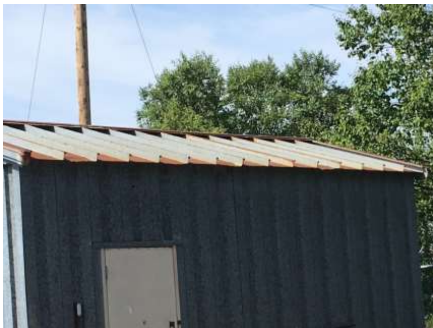
Surface corrosion on roofing panels.
