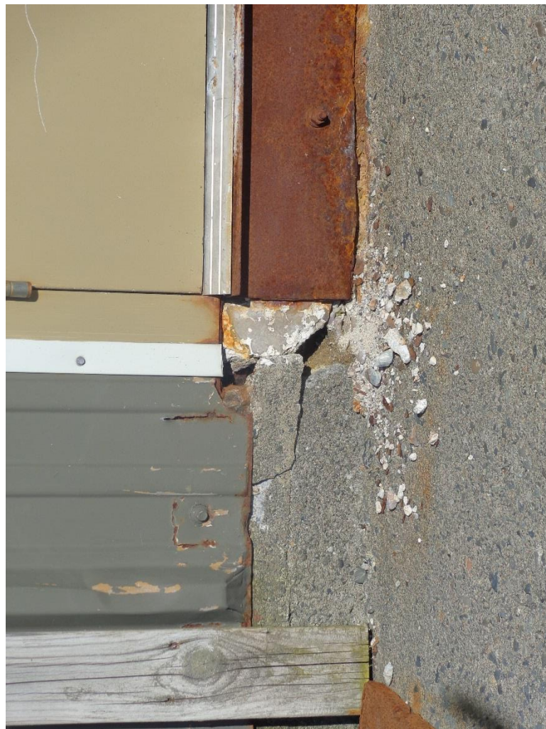
Photo 2 - Damage to Concrete Foundation Wall
