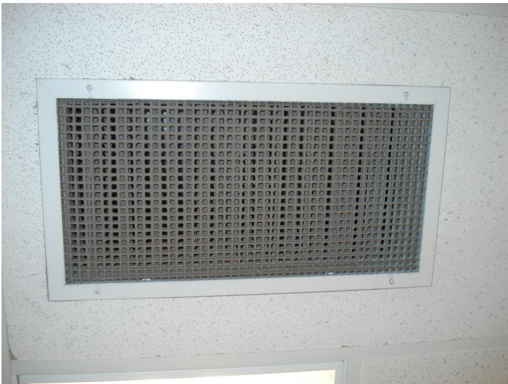
Photo 24 - Return Grilles Very Dirty
