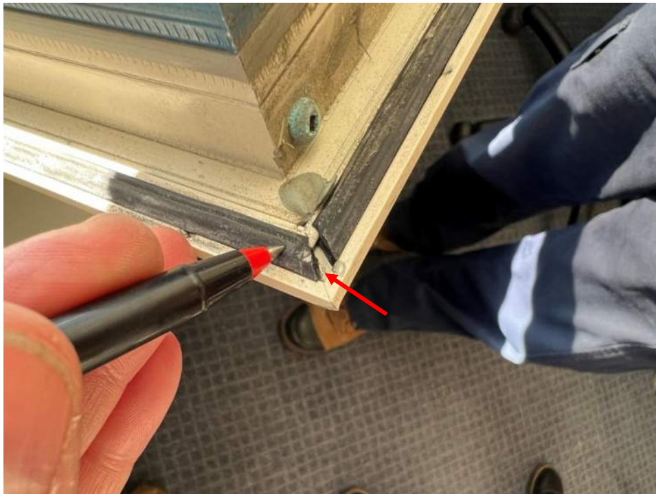
Photo No. 12: Typical view of weather stripping appears in poor condition with gaps
