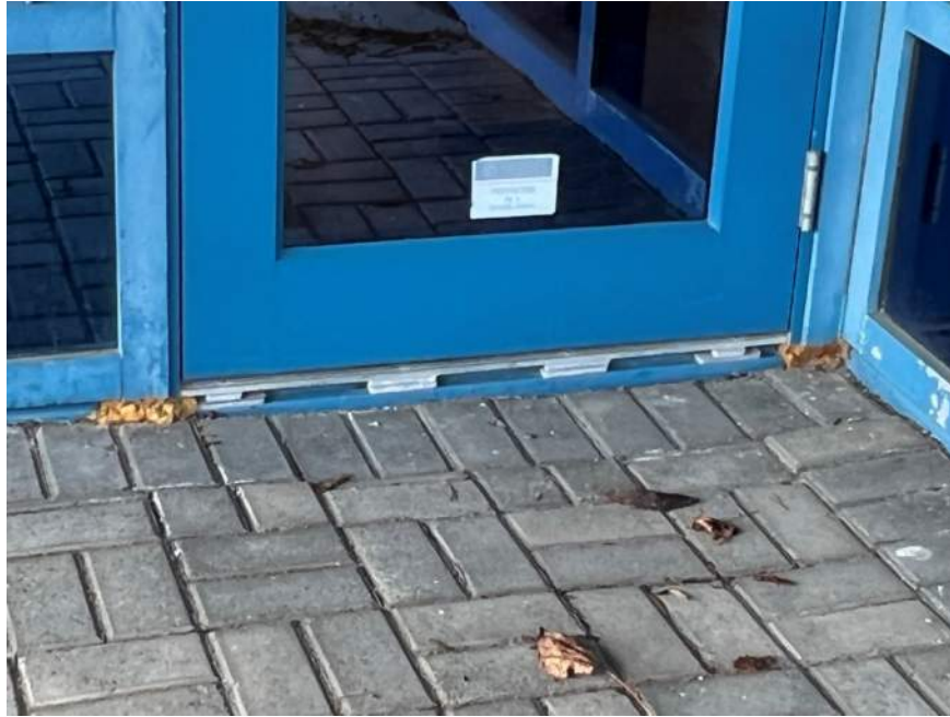
Photo No. 25: Typical view of aluminum storefront doors with exposed aluminum shims
