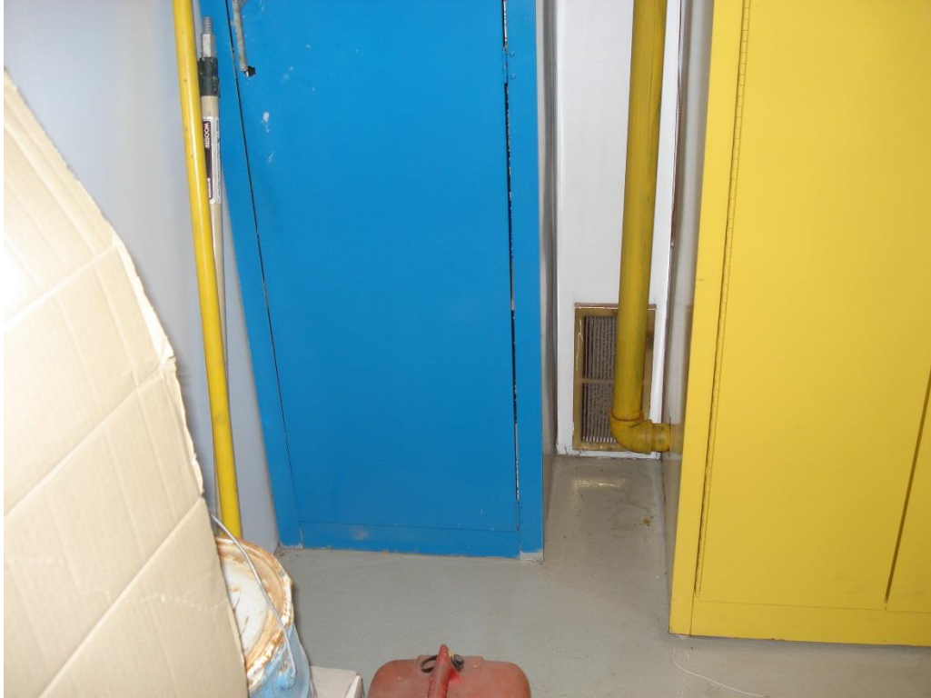
Photo 39 - Paint Storage Exhaust Air Grille and Ducting
