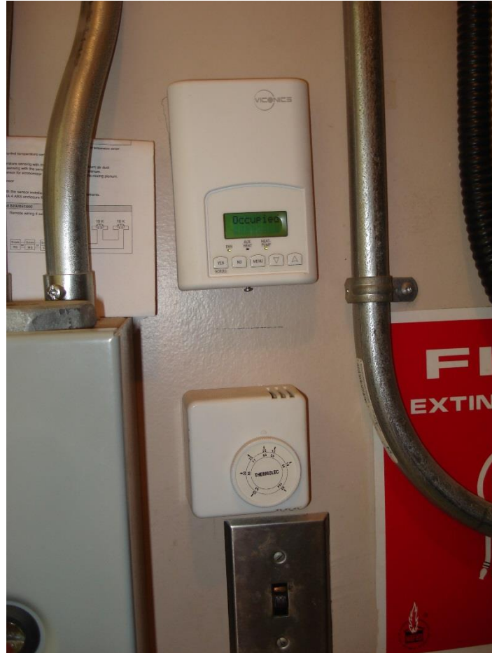
Photo 22 - Main System Controller
