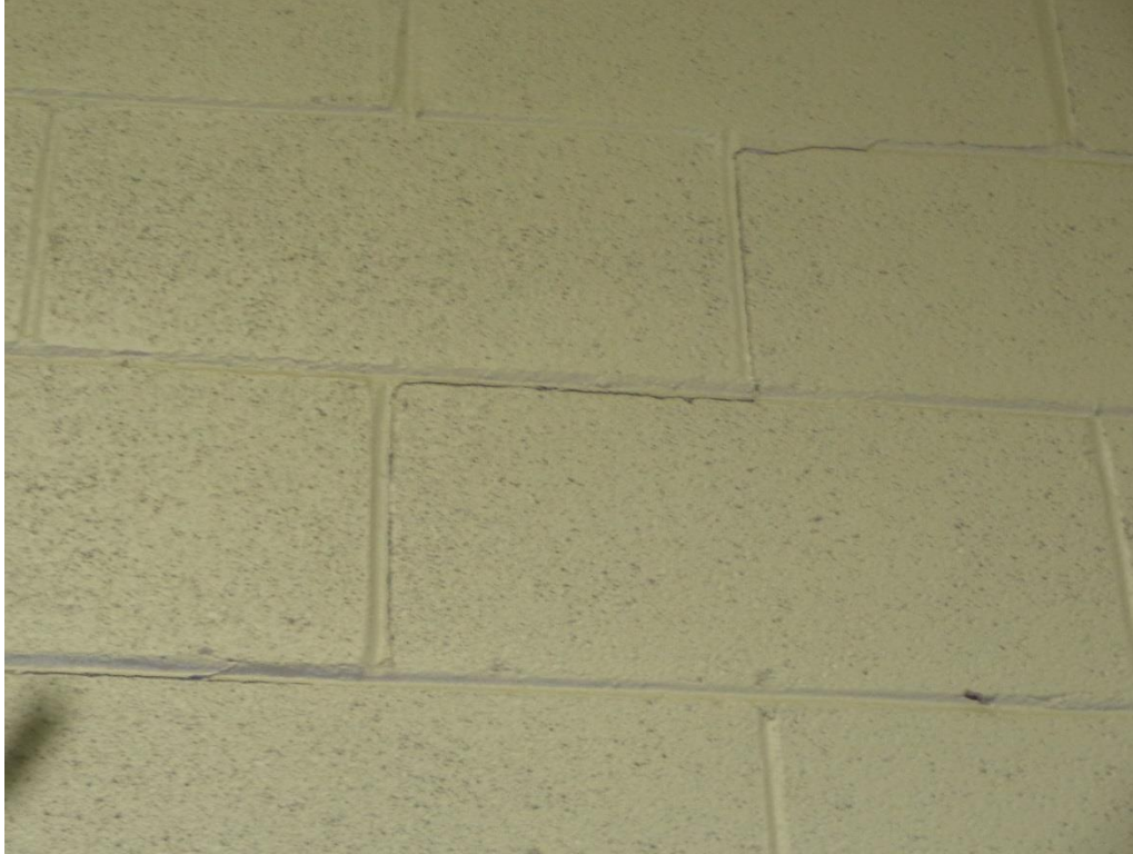
Photo 13 - Settlement Cracks in Block Wall (2)
