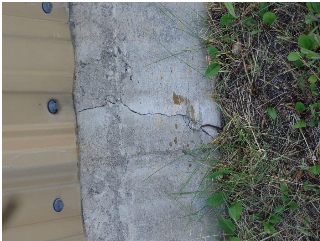
Photo 1 - Vertical Crack in Foundation Wall
