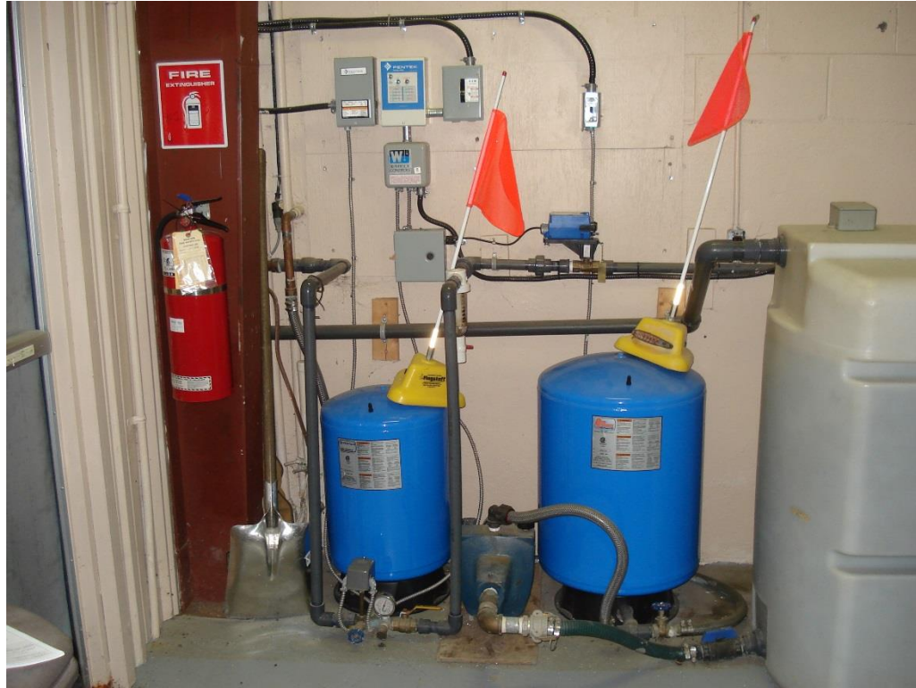
Photo 7 - Domestic Water Pressure Tanks and Piping
