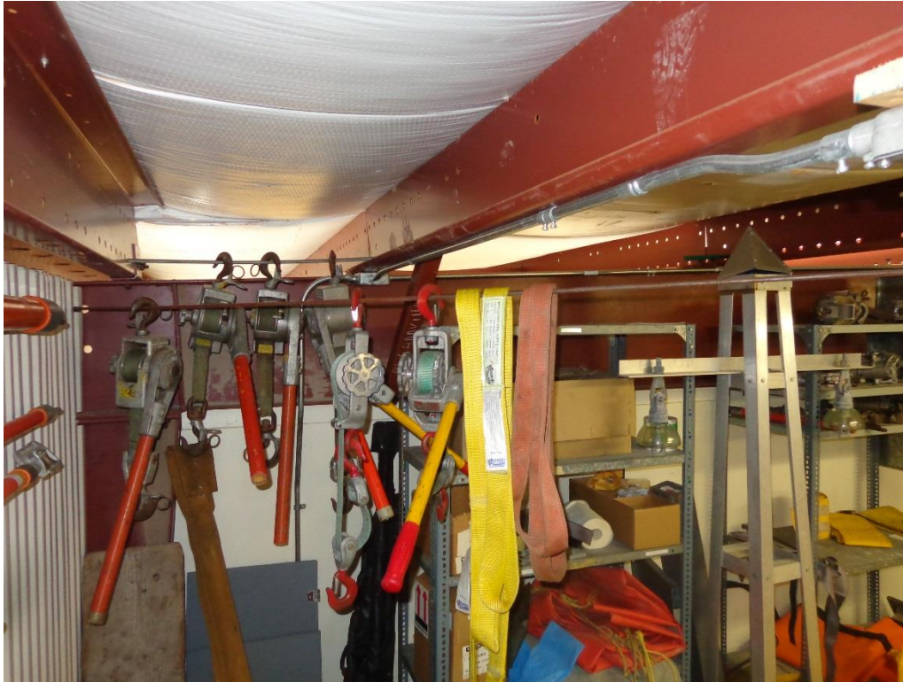
Photo 9 - Equipment Hung from Steel Tie Rod
