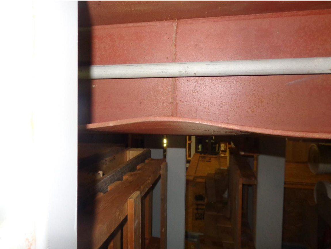
Photo 11 - Deformation in Column due to Impact (3)
