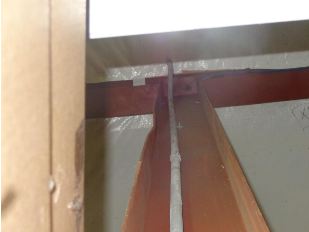
Photo 9 - Deformation on Column Due to Impact (1)
