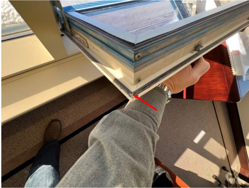
Photo No. 13: Typical view of weather stripping appears in poor condition (red arrow)
