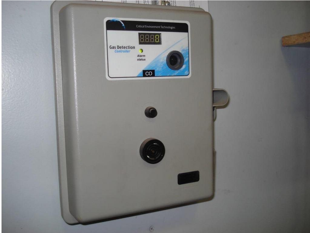
Photo 9 - CO Gas Detection System
