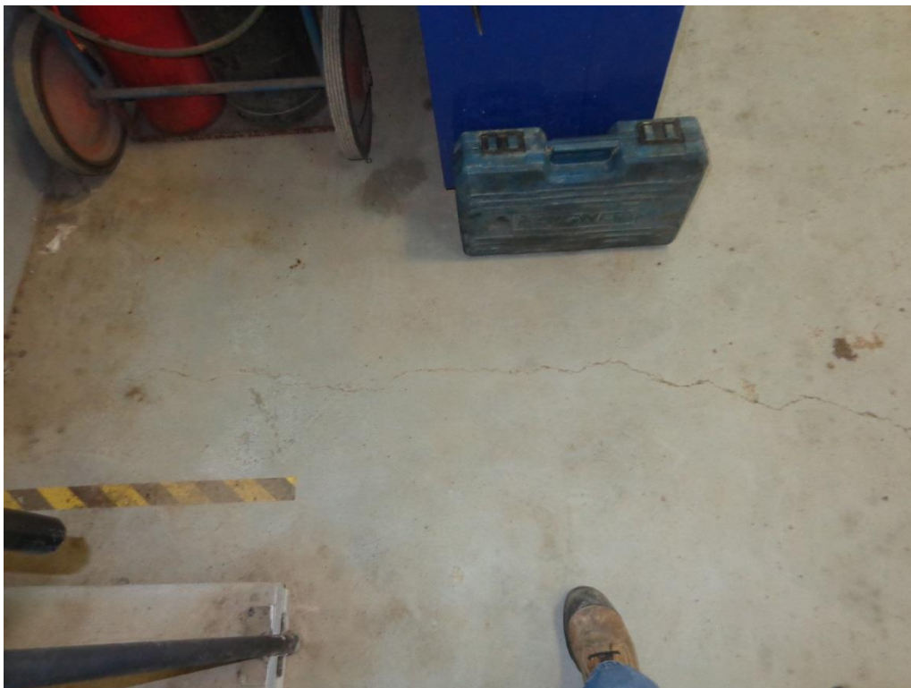
Photo 4 - Shrinkage Crack in Garage Interior Slab
