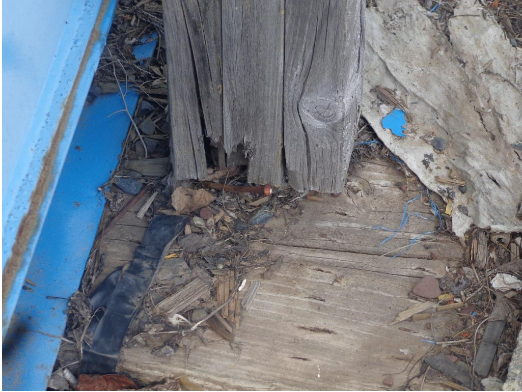
Photo 23 - Rotting Post of Equipment Platform
