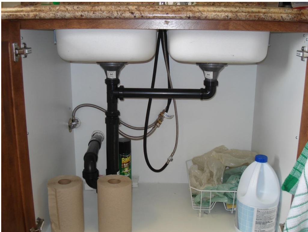
Photo 2 – ABS Waste Piping
