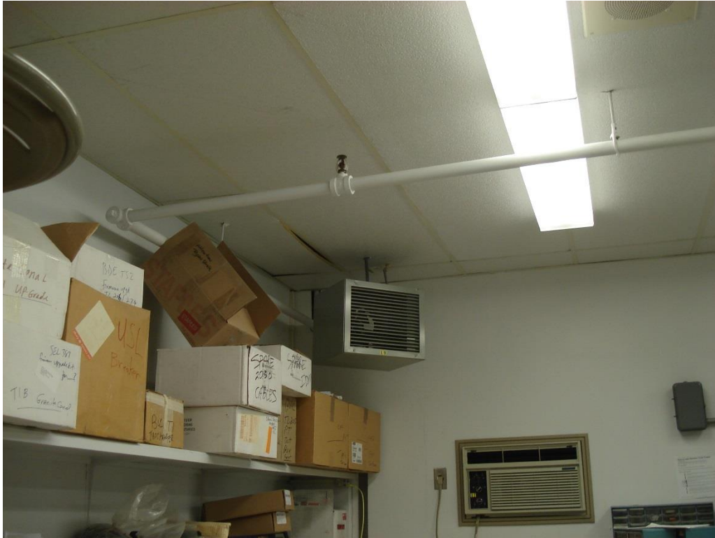
Photo 31 - Workshop Wall AC Unit
