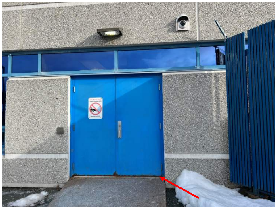
Photo No. 24: Typical view of rust formation at the bottom of the doors (red arrow)
