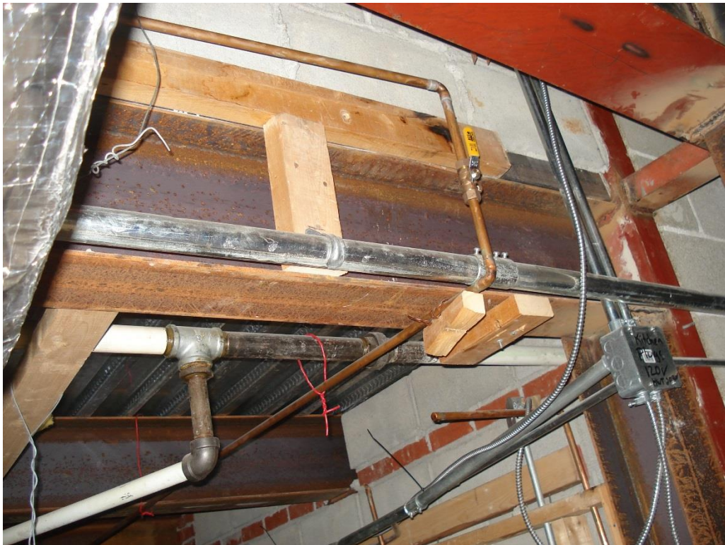
Photo 8 - Water Piping Not Properly Supported
