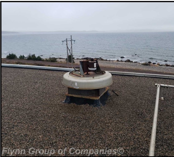
pump house #1: View of area of missing hood from fan unit to be addressed
