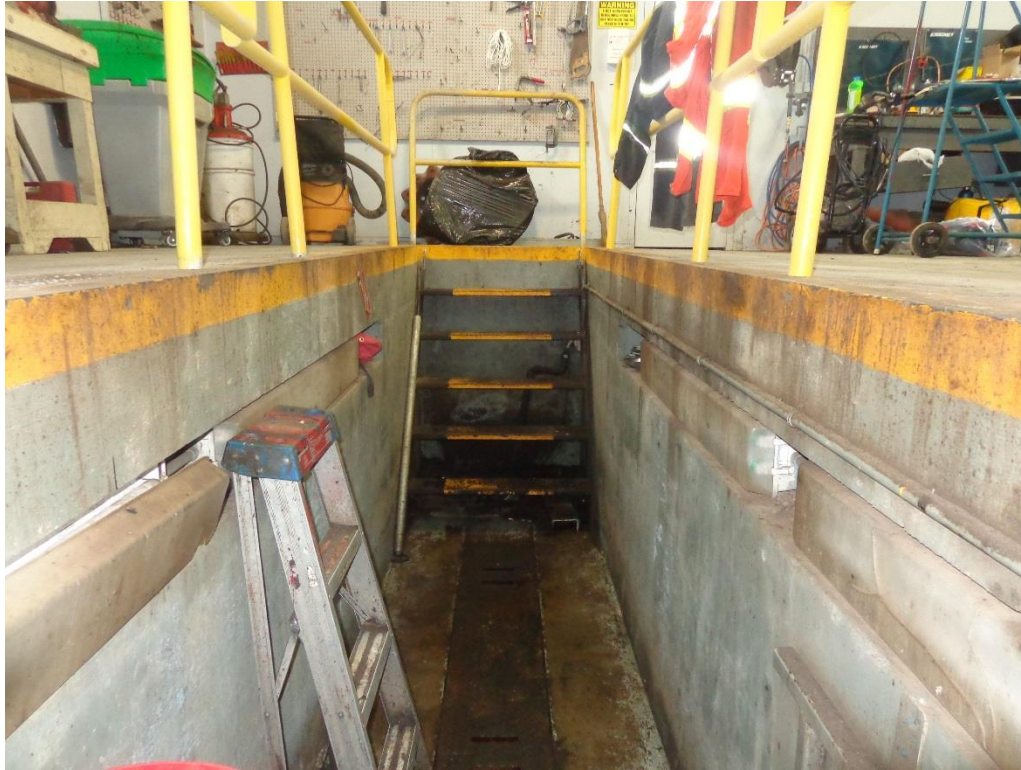
Photo 23 - Service Pit Staining
