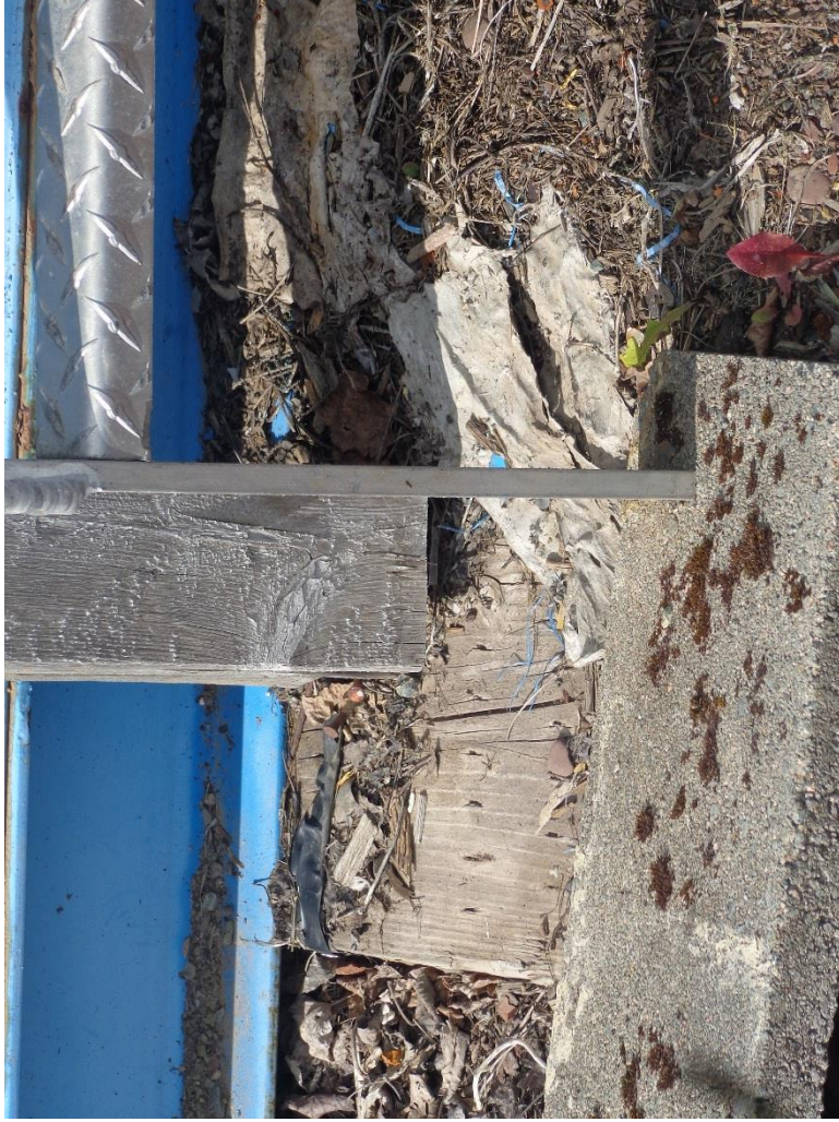
Photo 22 - Post Not Bearing on Ground
