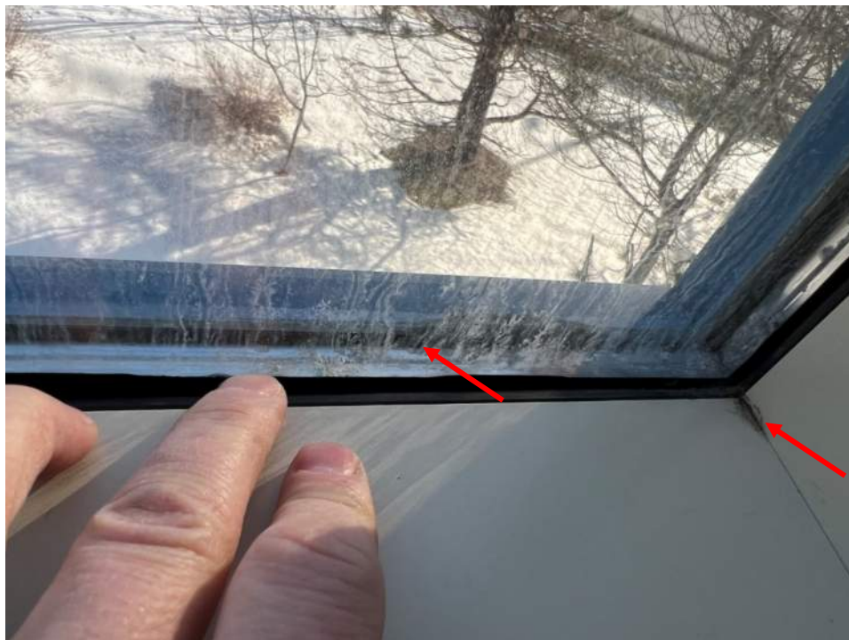
Photo No. 8: Typical view of curtain wall is in fair-to-poor condition overall (red arrows)
