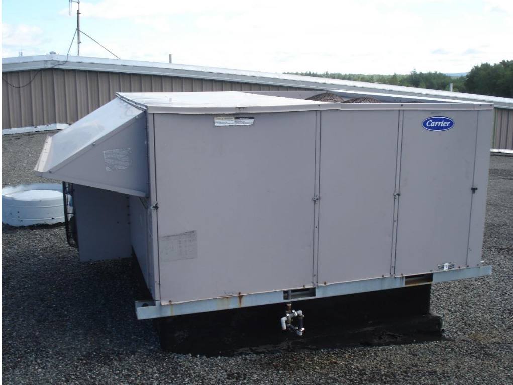
Photo 21 - Office Area Rooftop AC Unit
