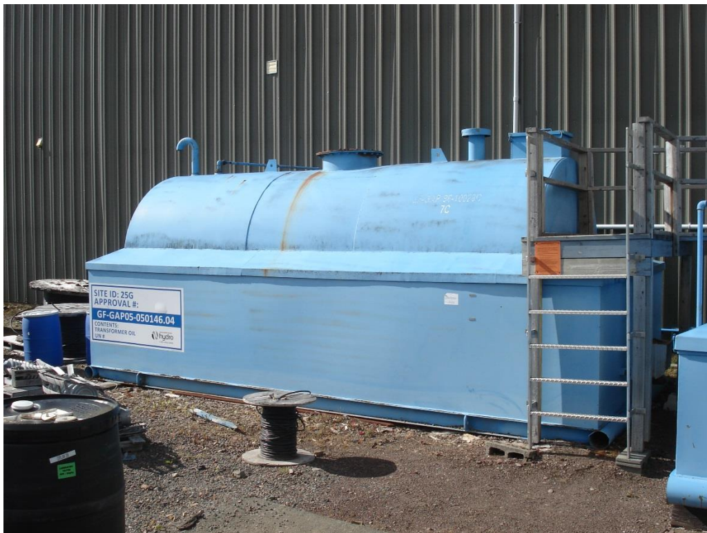
Photo 14 – 18,000 L Transformer Oil Tank (Used Oil)
