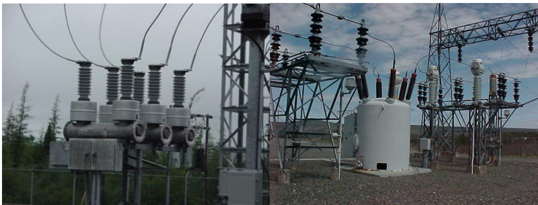
Figure 9: Oil Circuit Breakers (Left) and SF 6 Circuit Breakers (Right)
