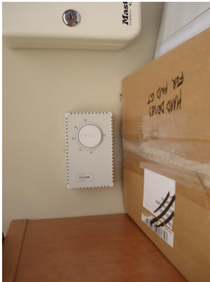
Photo 26 – Office Area Zone Thermostat
