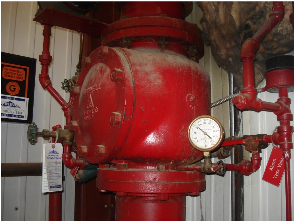
Photo 44 - Wet Sprinkler System Alarm Valve
