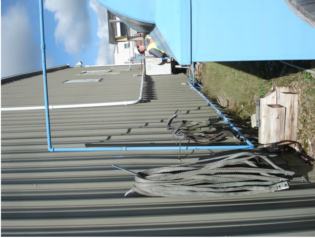
Photo 18 - Tank Piping Not Properly Supported
