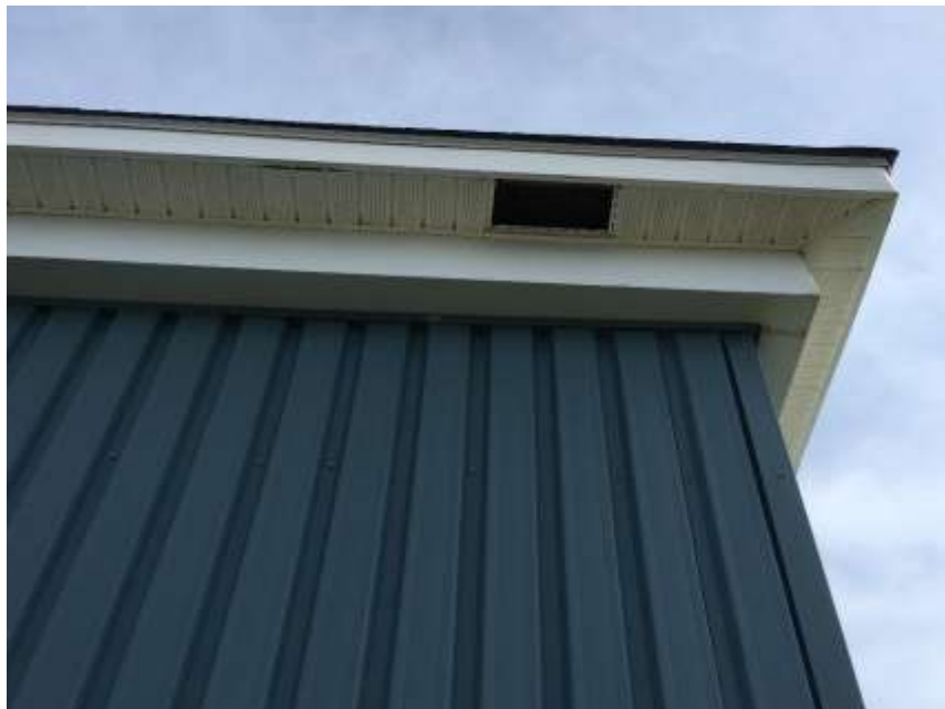
Soffit/fascia of double roof with unprotected soffit hole.
