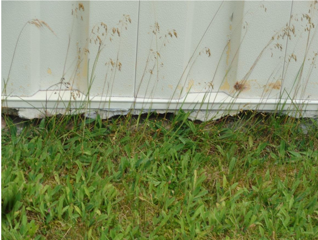
Photo 3 - Large Spall in Foundation
