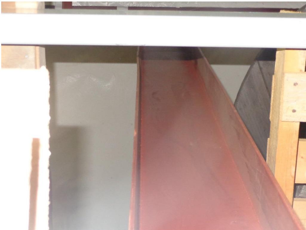
Photo 10 - Deformation in Column due to Impact (2)
