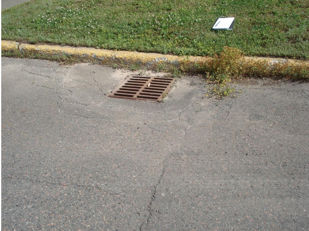
Photo 11 - Catch Basin Not Up To Grade
