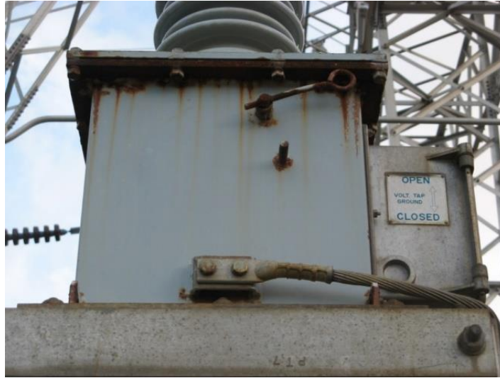
Figure 2: Rusting Potential Transformer
