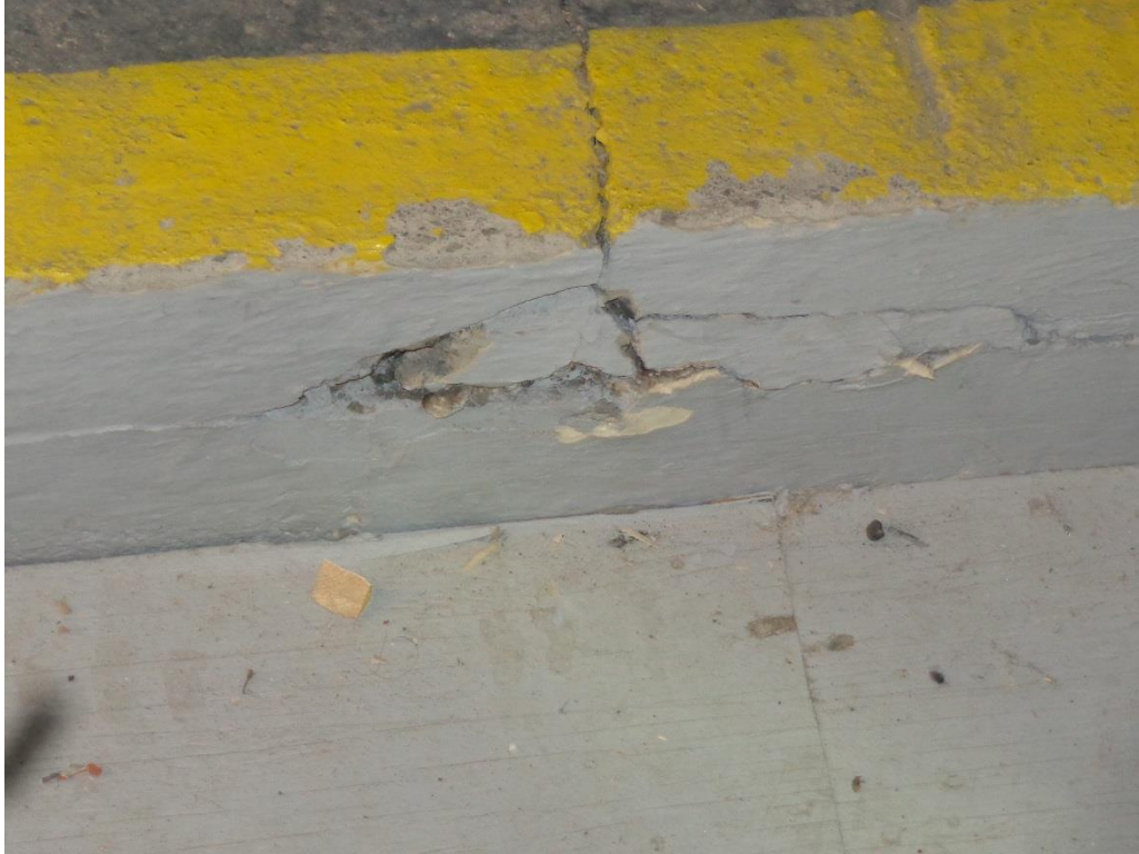
Photo 17 - Horizontal Crack in Slab
