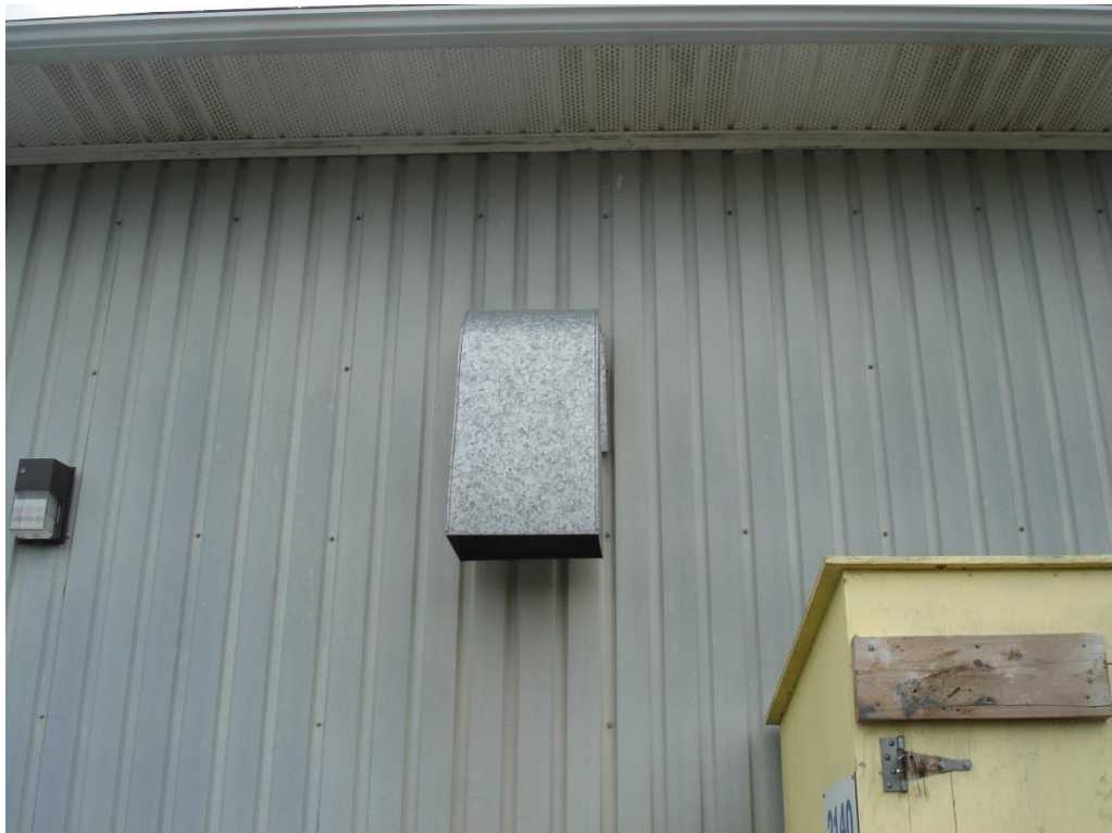
Photo 6 - Garage Exhaust Fan Hood
