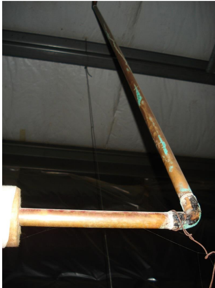
Photo 10 - Uninsulated Domestic Water Piping
