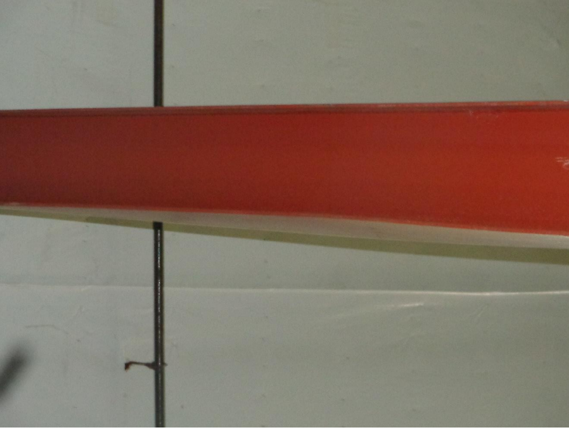
Photo 12 - Twist in Column Possibly Due to Overstress (1)
