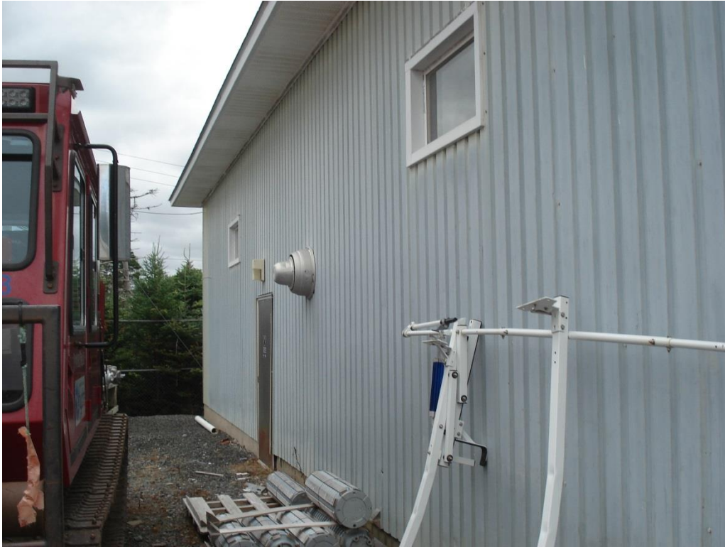
Photo 7 - Service Pit Sidewall Exhaust Fan
