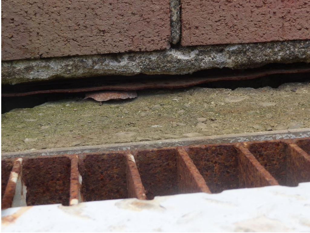
Photo 19 - Shelf Angle in Poor Condition
