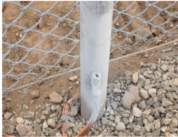
Figure 7: Typical Grounding Connection on Terminal Station Fence
