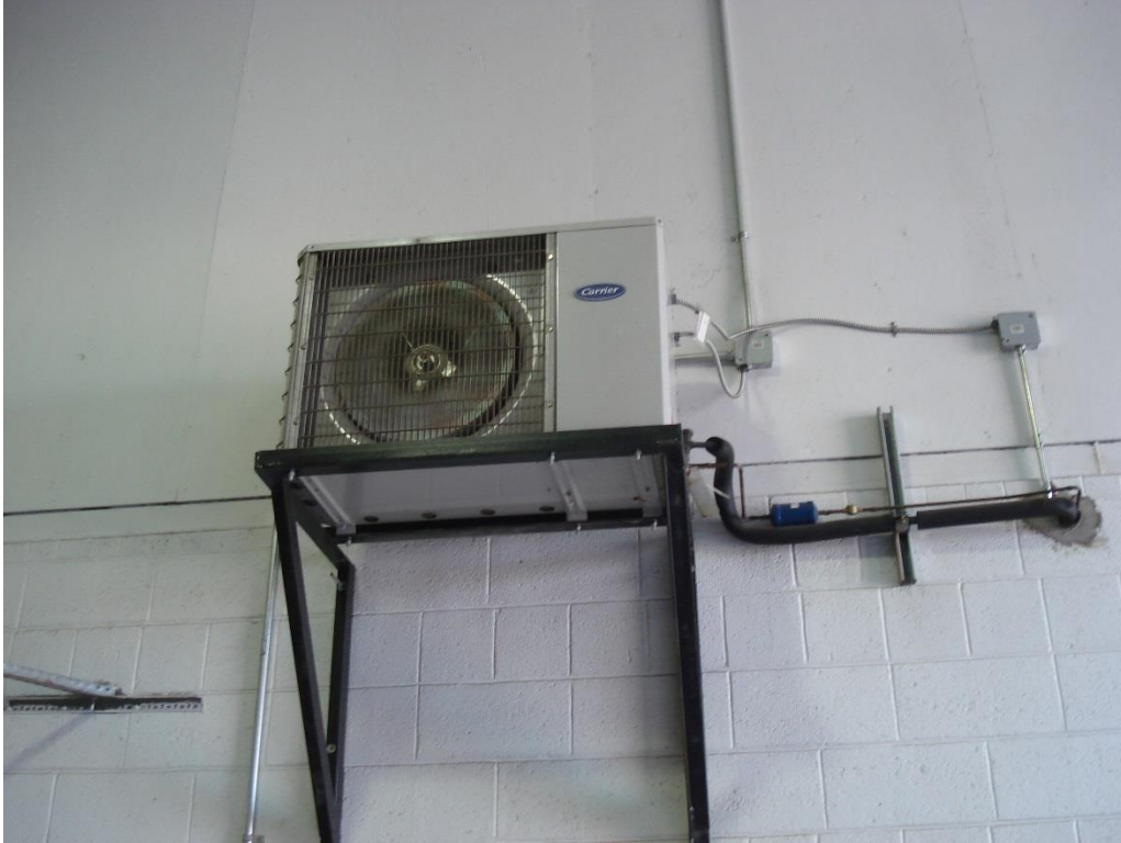
Photo 25 - Server Room Condenser Unit
