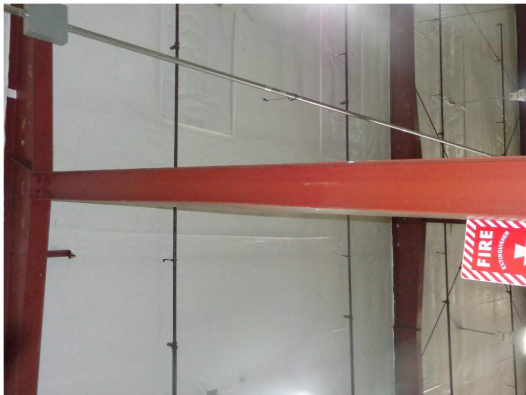
Photo 13 - Twist in Column Possibly Due to Overstress (2)
