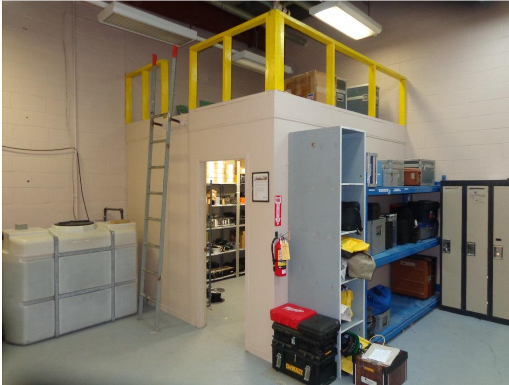
Photo 11 - Mezzanine in Telecontrol Room
