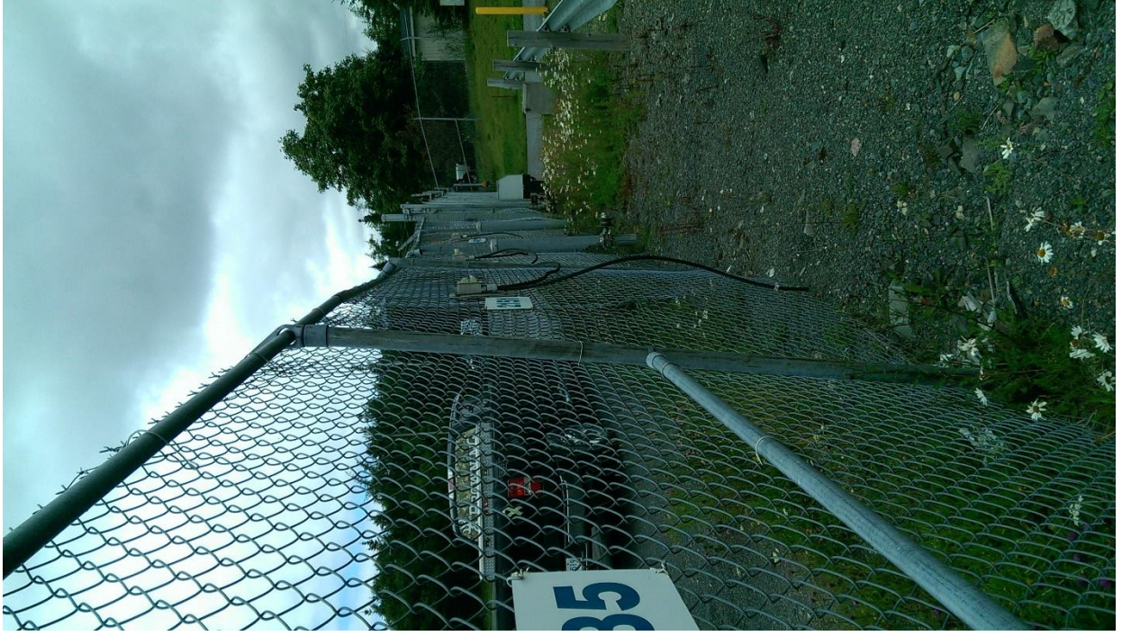
Photo 18 - Top Brace Bent and Fence Leaning
