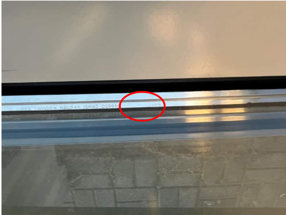
Photo No. 5: Typical view of a 1989 IGU date stamp (red circle)
