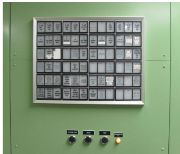
Figure 19: Annunciator Commonly Found in Hydro Terminal Stations
