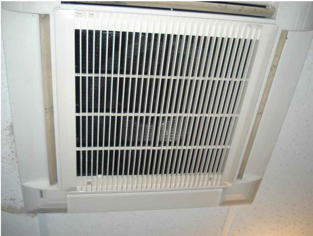
Photo 26 - Server Room Evaporator Unit
