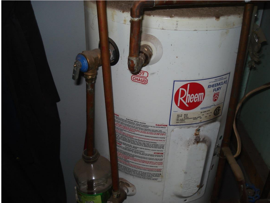
Photo 5 - Hot Water Tank
