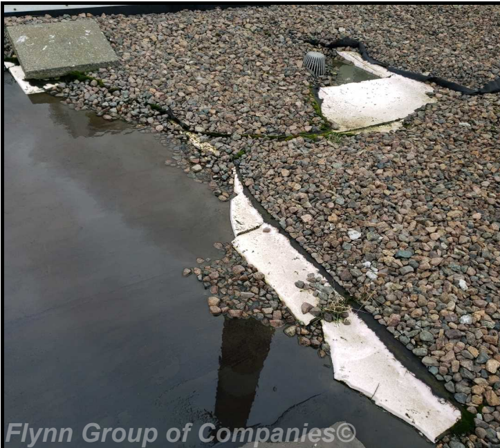
pump house #2: Area of wind swept ballast at corner of building
