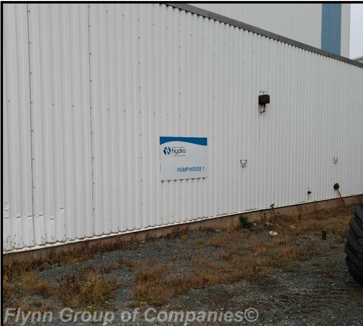
Front of Building: View of pump house #1
