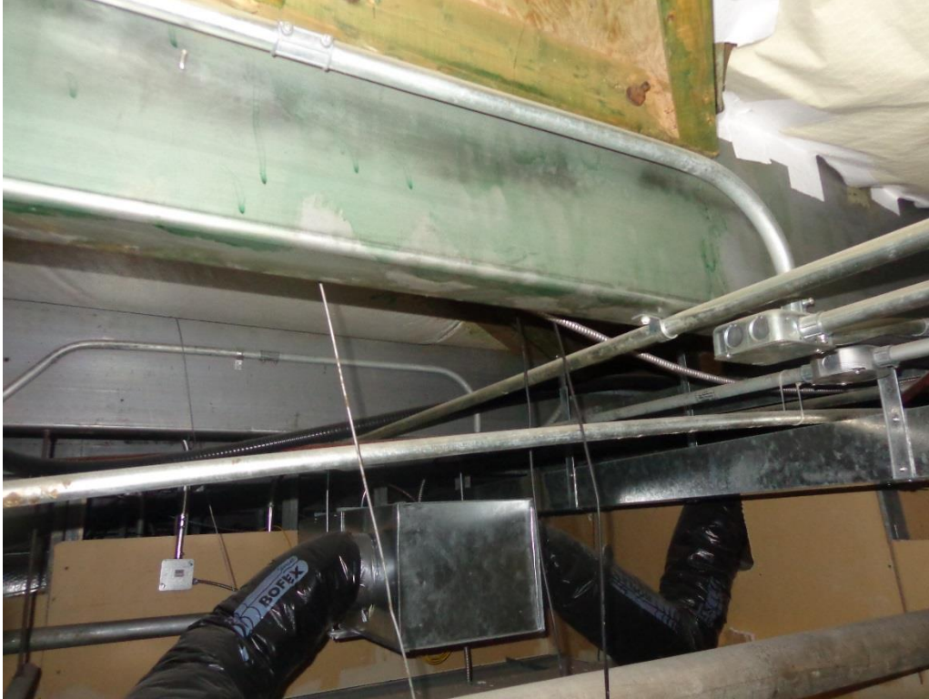
Photo 21 - Typical Bypass Terminal Unit
