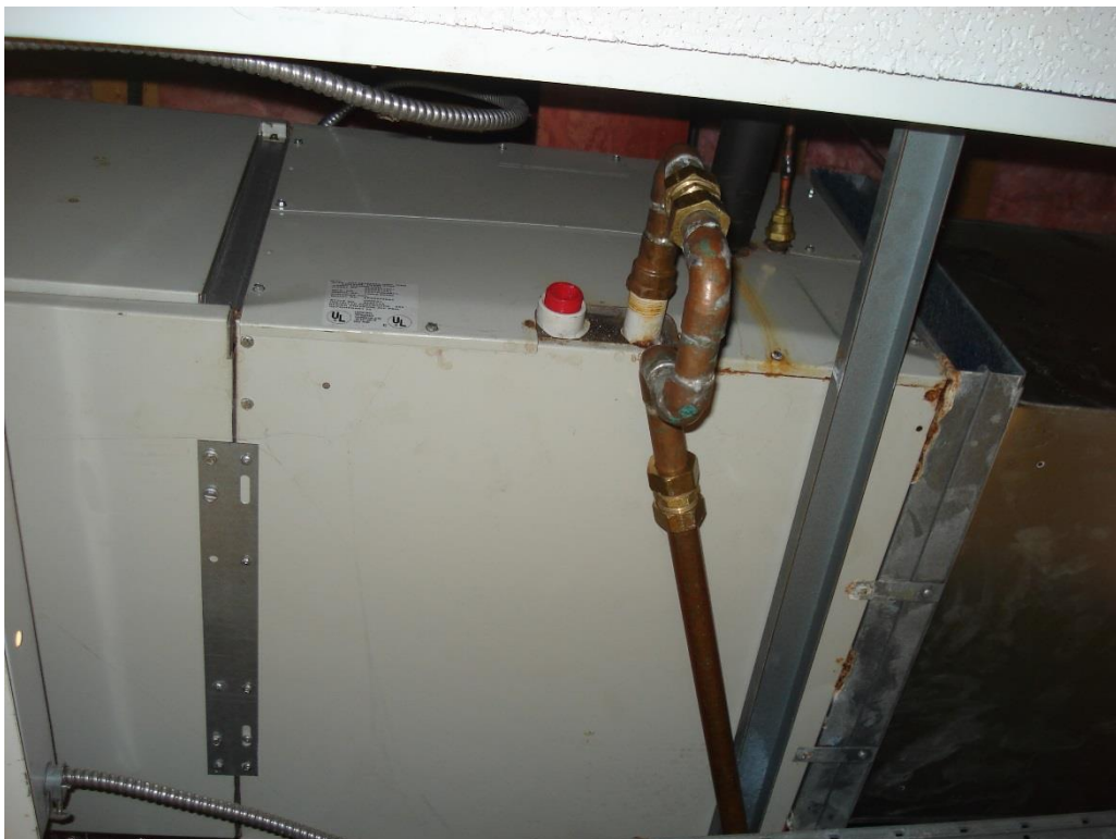
Photo 30 - Transformer Shop Offices Evaporator Unit
