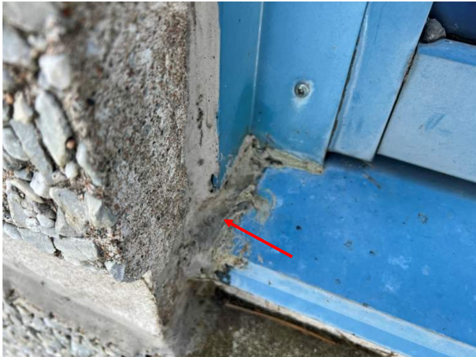
Photo No. 26: Typical view of sealant in poor condition (red arrow)
