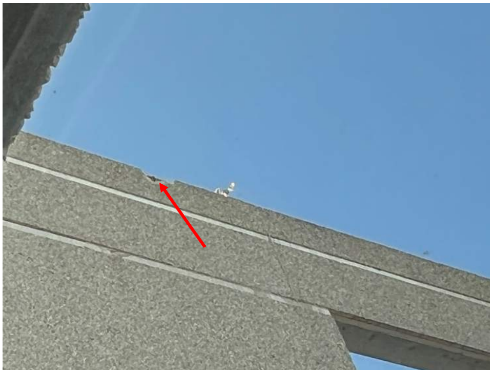
Photo No. 22: View of the precast panel surfaces was noted to be peeling or failing (red arrow)
