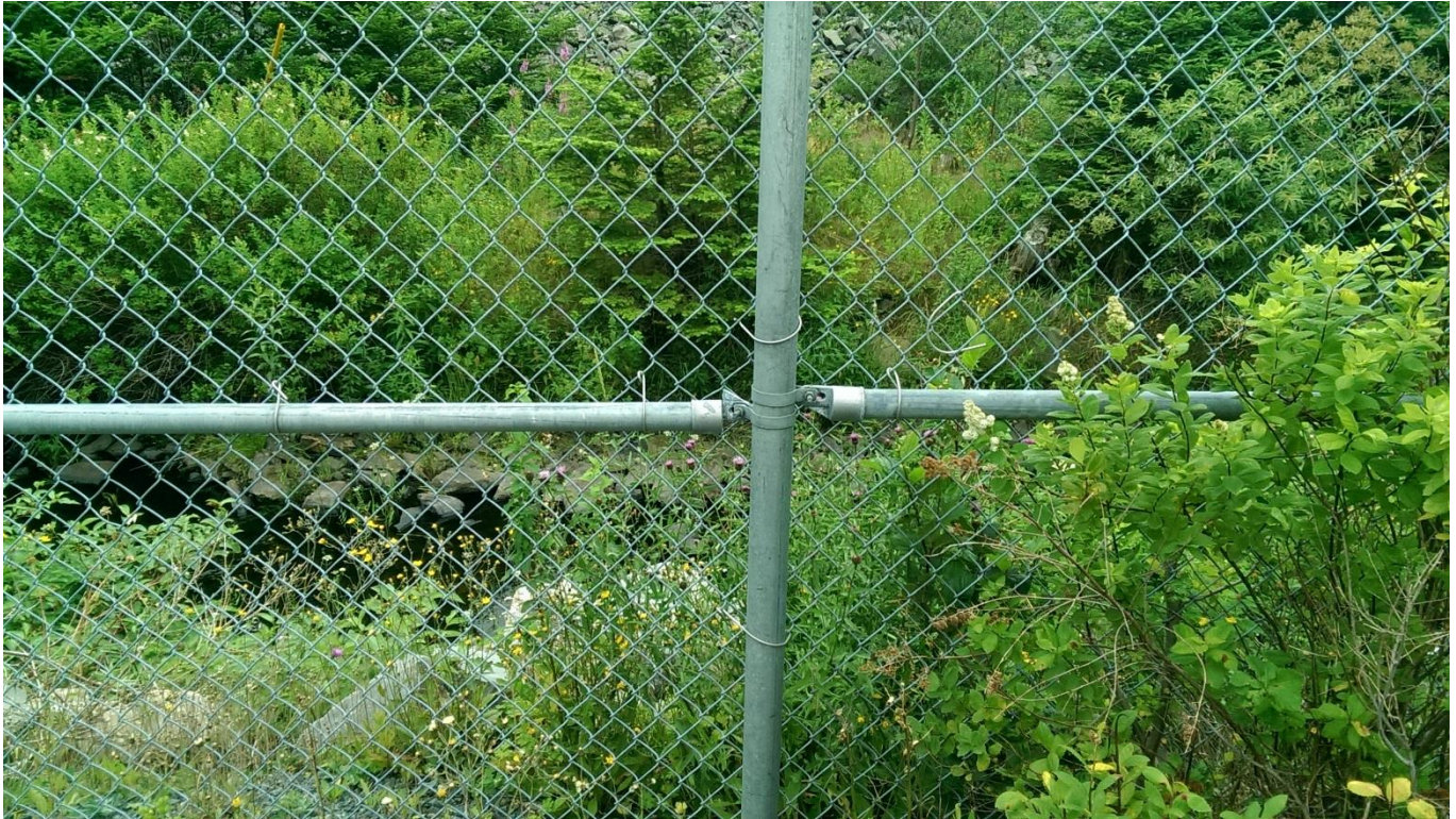
Photo 15 - Brace Fitting Broken
