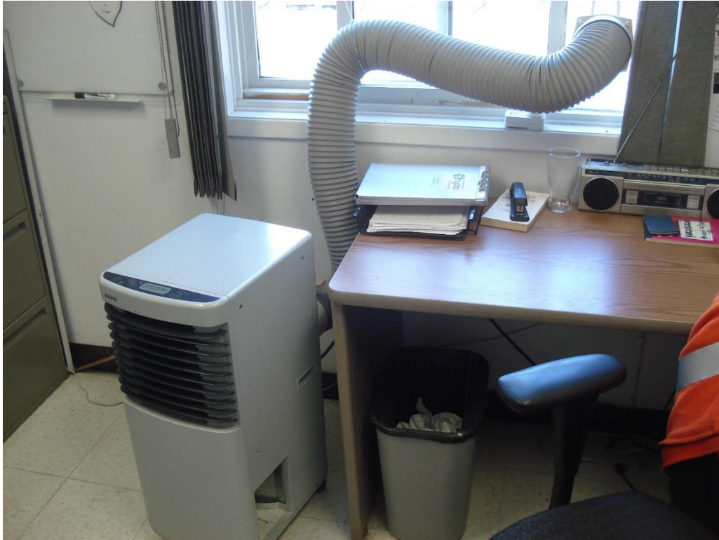
Photo 29 - Portable Air Conditioning Unit
