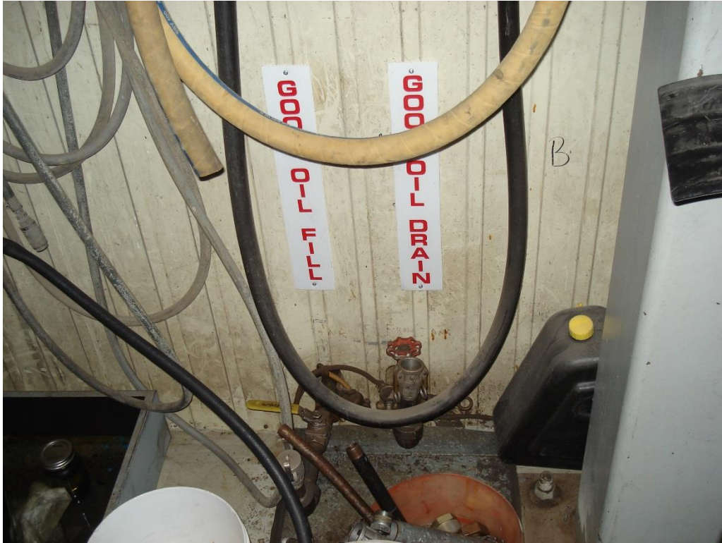
Photo 19 – Transformer Oil Supply and Fill Pipes
