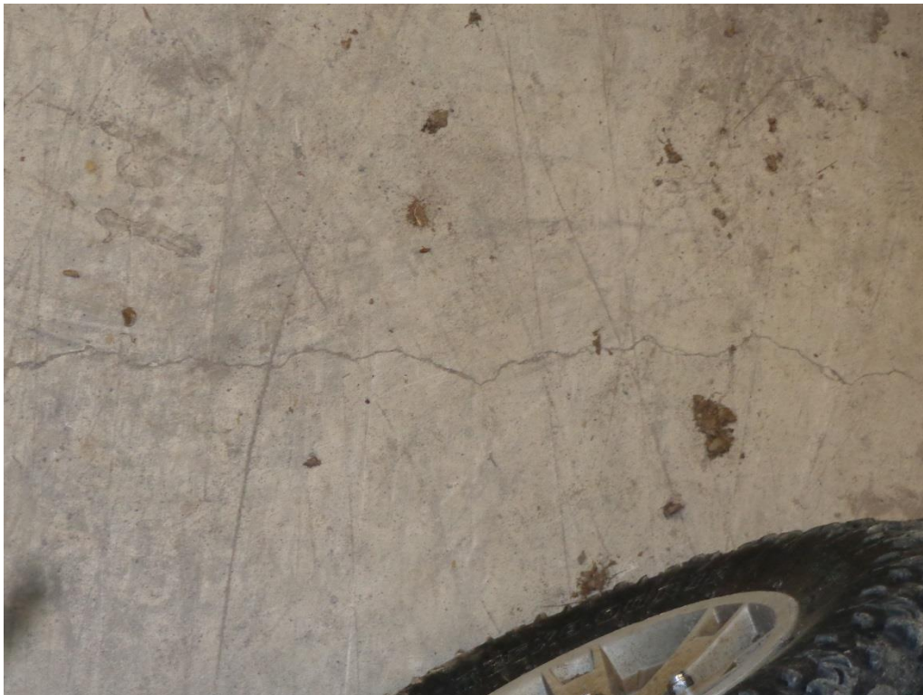
Photo 2 - Floor Shrinkage Cracks
