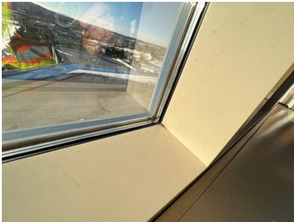
Photo No. 10: Typical view of curtain wall is in fair-to-poor condition overall
