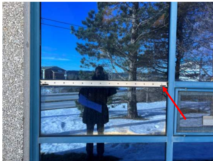
Photo No. 16: Typical view of pressure plates that have been installed upside down (red arrow)
