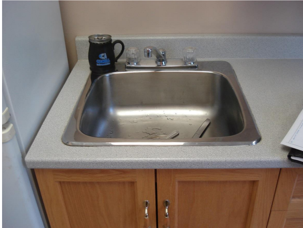
Photo 17 - Lunch Room Sink
