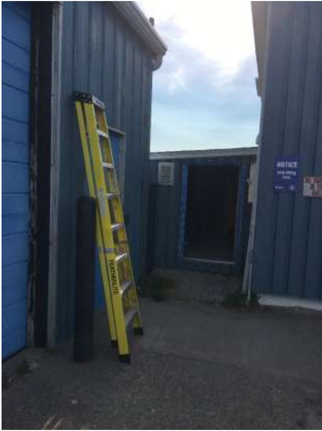
Proximity of lean-to flammable storage between main and storage buildings.
