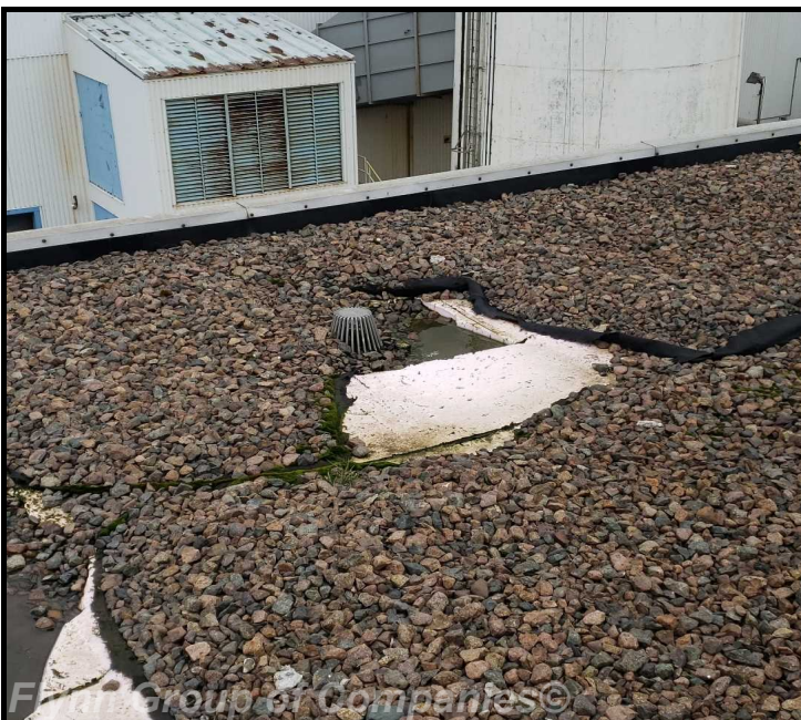
Section A: View of area of wind damage around one drain
