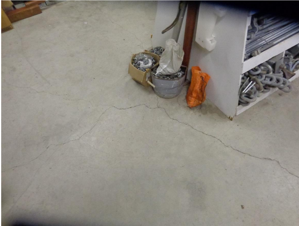
Photo 5 - Shrinkage Cracks in Interior Slab (2)
