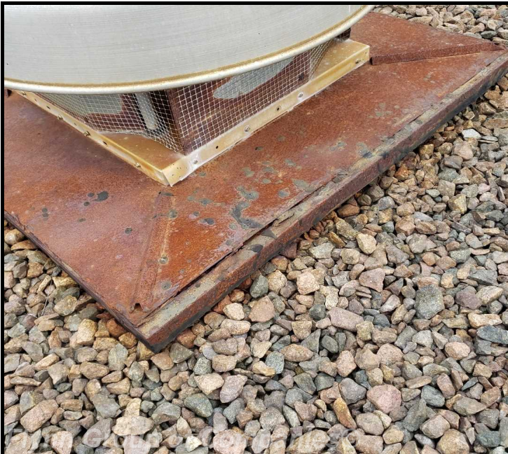
pump house #2: View of area of open seams around fan curb top
