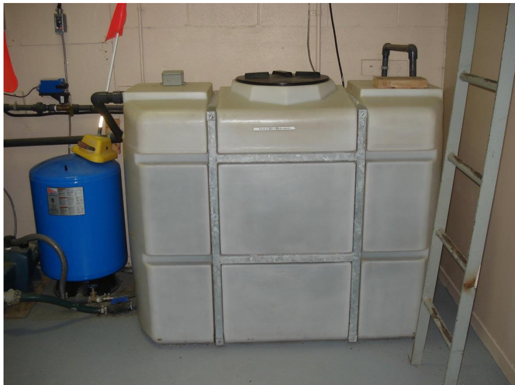
Photo 8 - Domestic Water Storage
