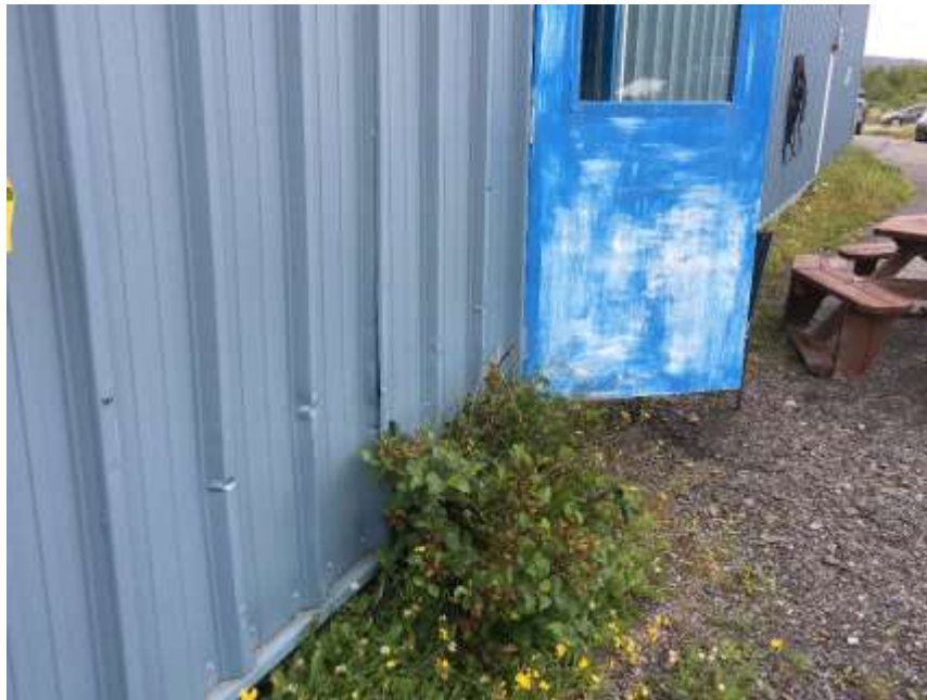
Left façade kitchen door and cladding damage.
