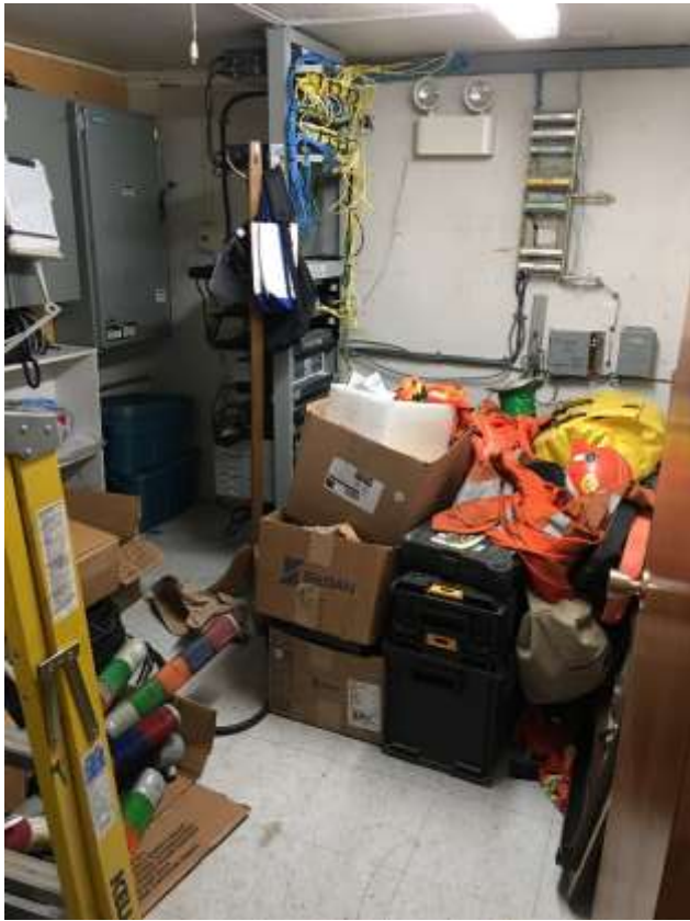
Electrical/ communications room. Note items stored hazard.
