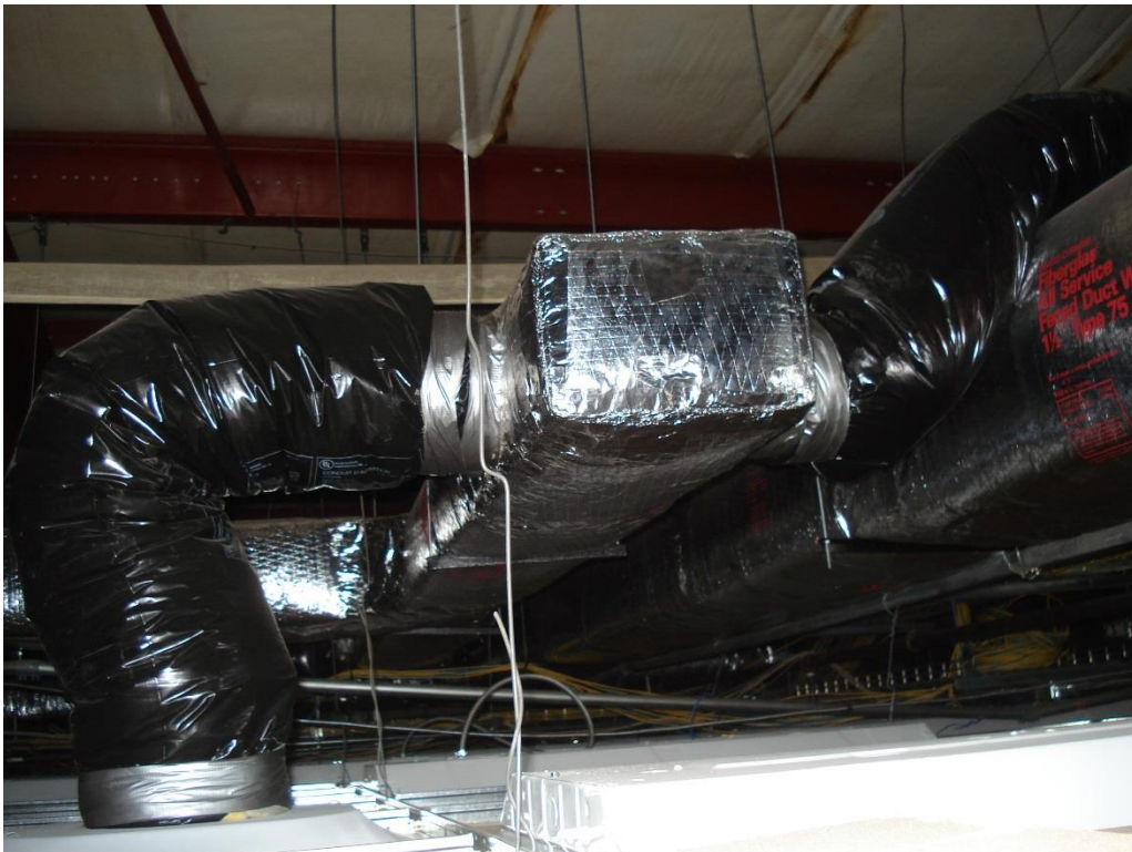
Photo 22 - Insulated Supply Ductwork
