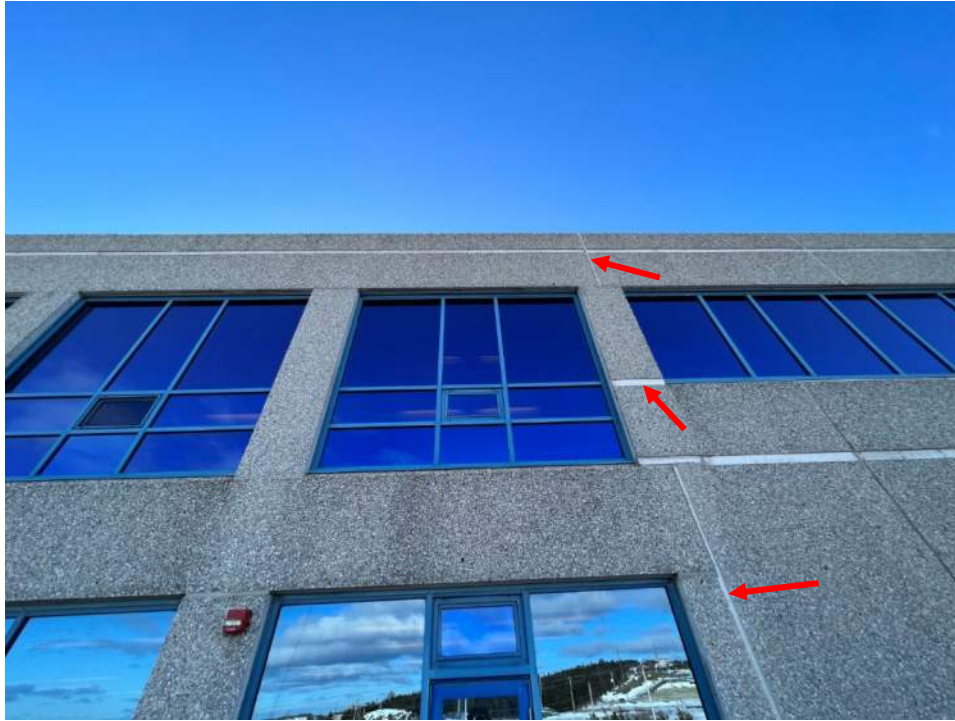
Photo No. 19: View of the localized precast panel joints has been repaired (red arrows)
