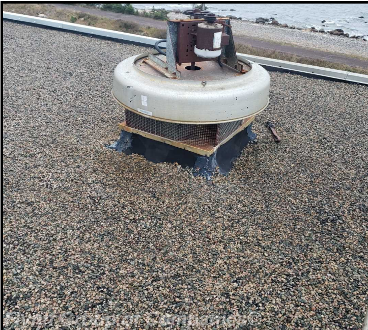
pump house #1: Areas of detail flashing in need of some sealant
