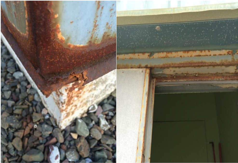
Figure 17: Building Exterior Cladding and Exterior Doorways Displaying Severe Rusting and Deterioration
