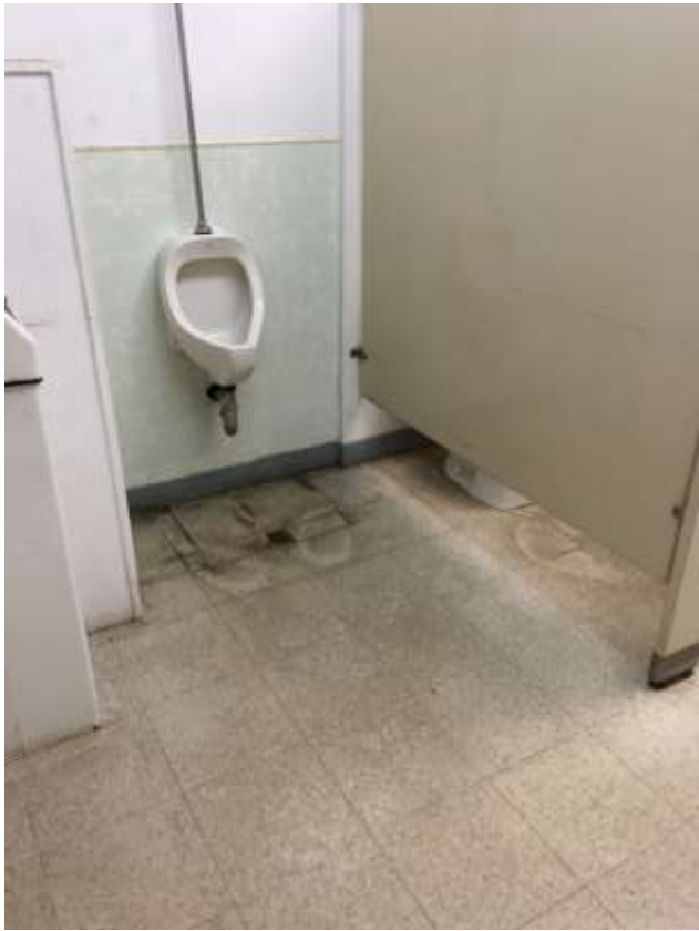
Male washroom. Note flooring condition.
