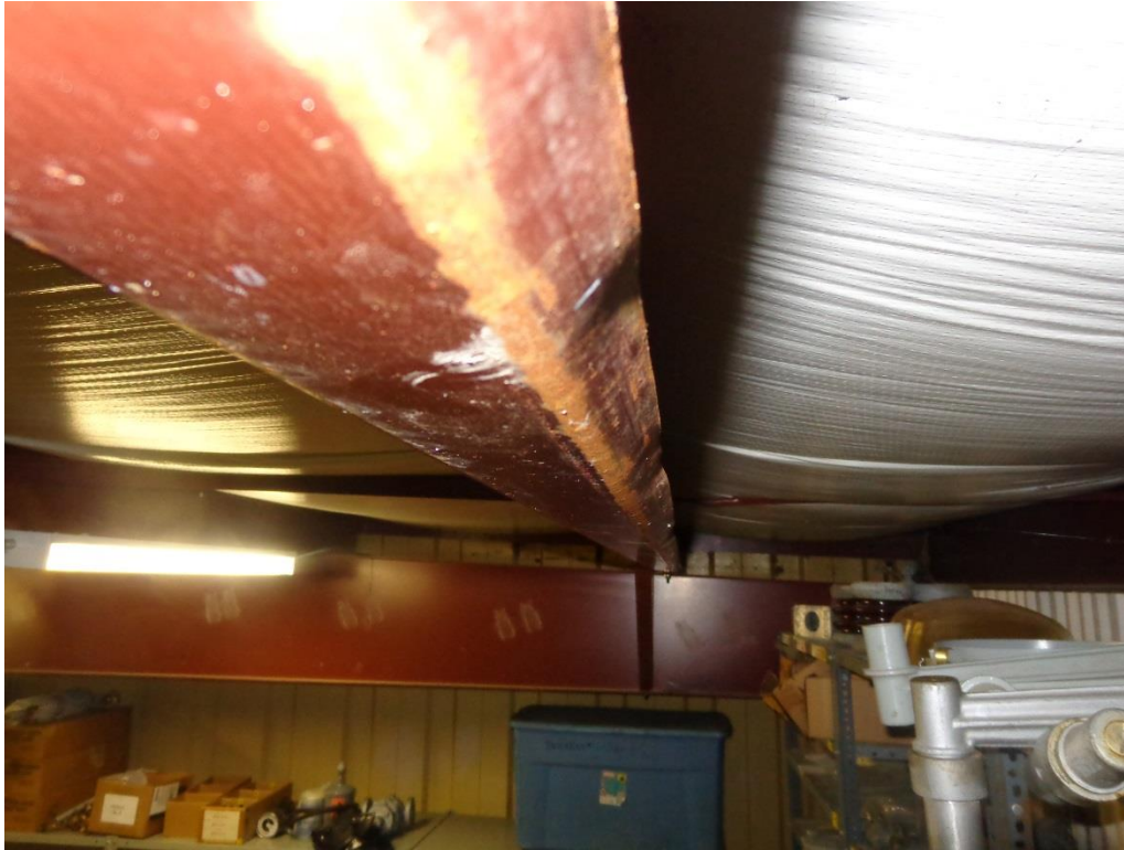
Photo 7 - Deformation of Purlin
