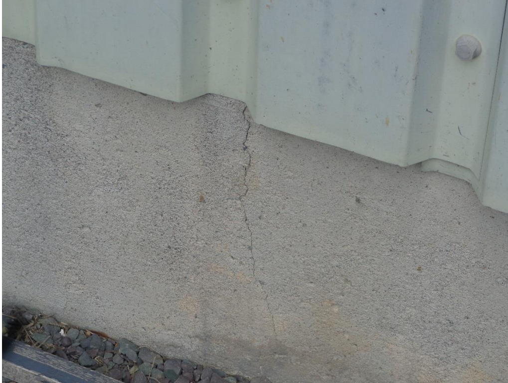
Photo 1 - Small Vertical Crack in Foundation Wall
