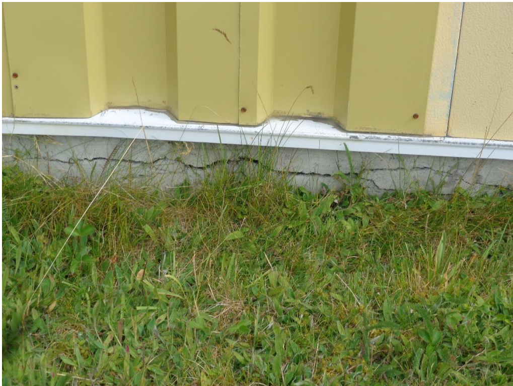
Photo 4 - Large Horizontal Crack in Foundation Wall
