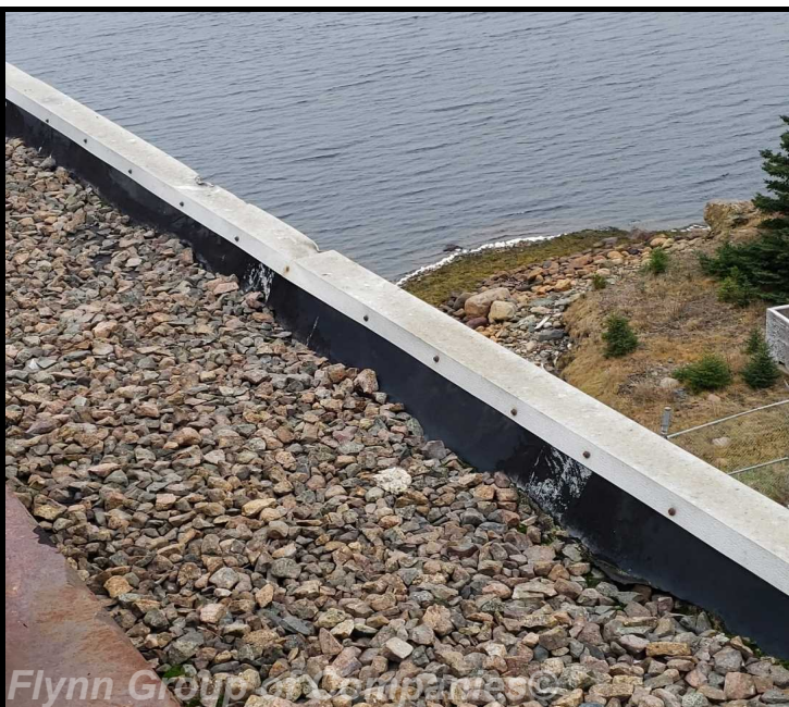
pump house #2: Areas of detail flashing with exposed mesh to be resealed
