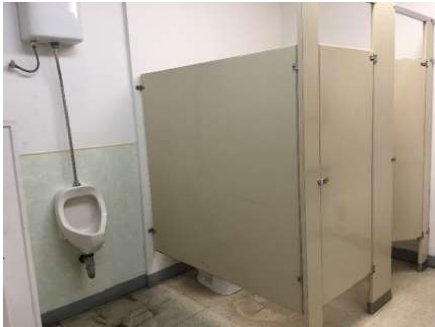
Male washroom. Note flooring condition.
