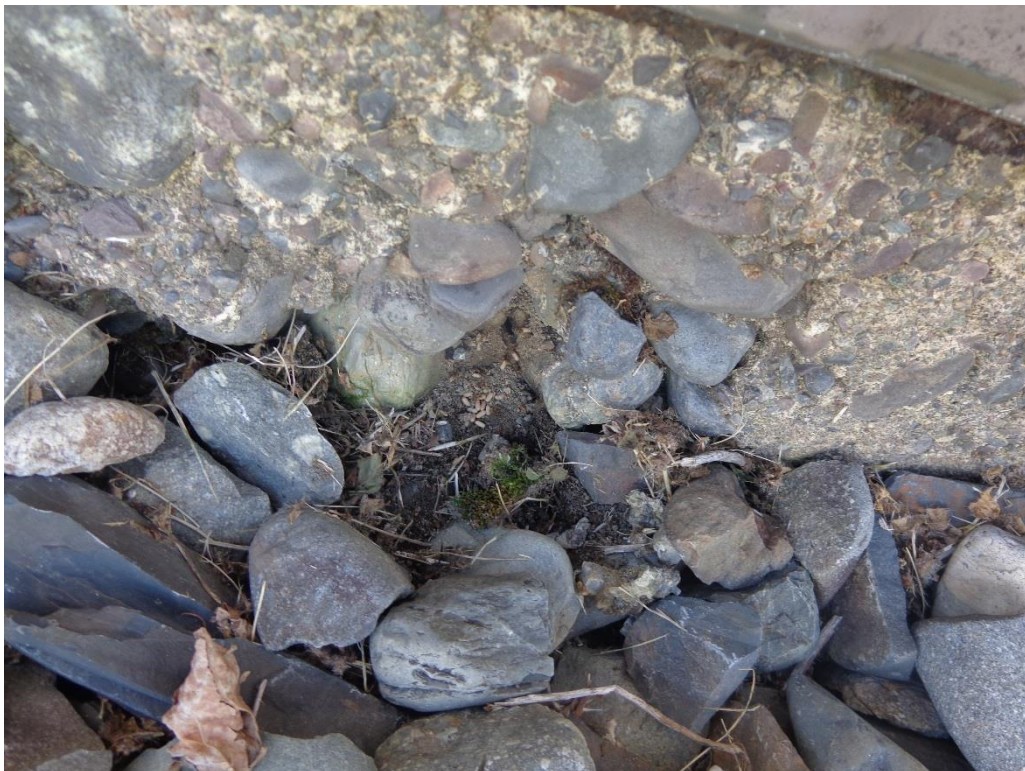
Photo 4 - Ants Entering Building Through Foundation Wall
