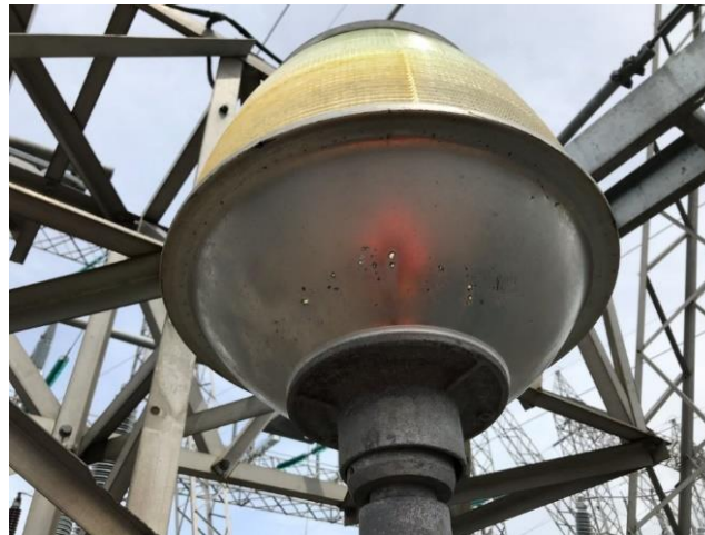
Figure 13: Light Fixture Showing Perforations due to Corrosion, Enabling Moisture Ingress
