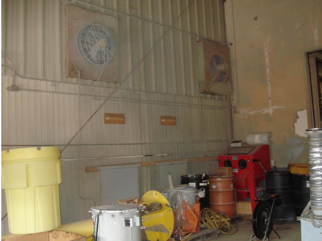
Photo 33 – Paint Room Propeller Exhaust Fans
