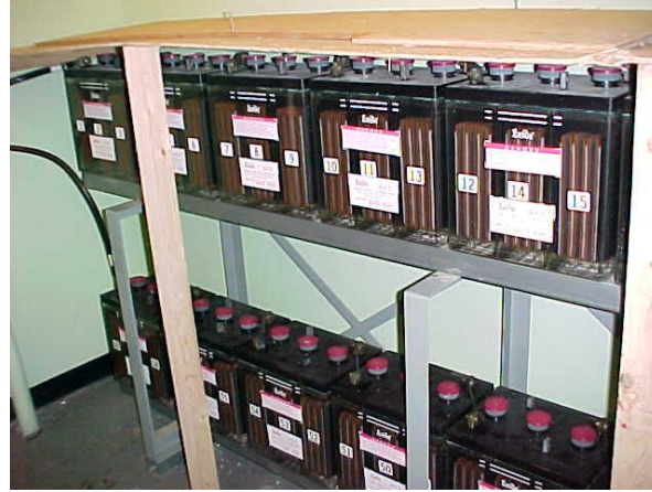
Figure 10: 125 Vdc Terminal Station Battery Bank
