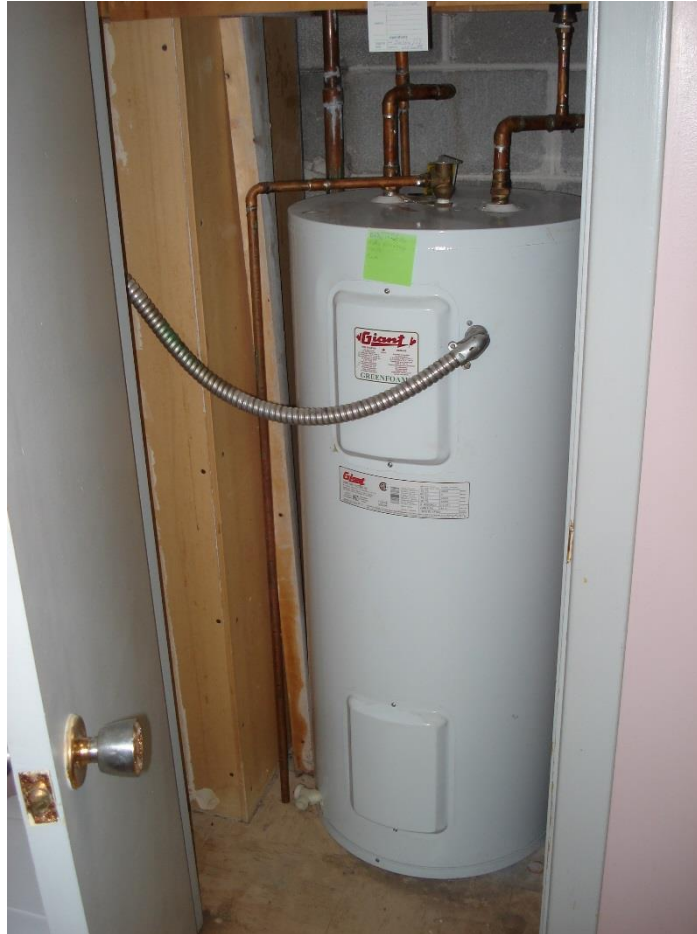
Photo 11 - Hot Water Tank
