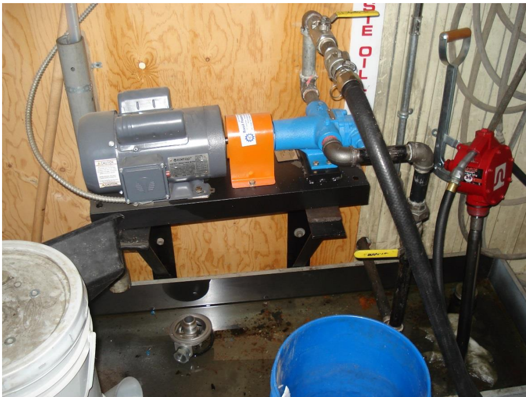
Photo 20 – Waste Oil Transfer Pump
