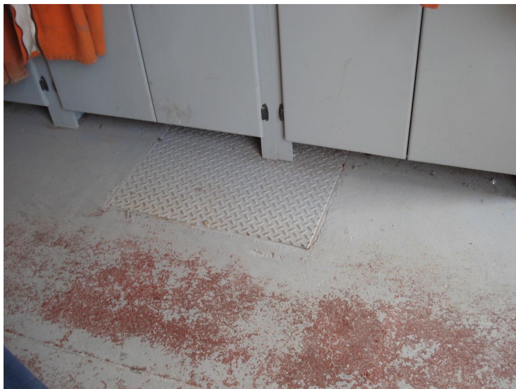
Photo 6 – Stabilizing Chamber Access Cover
