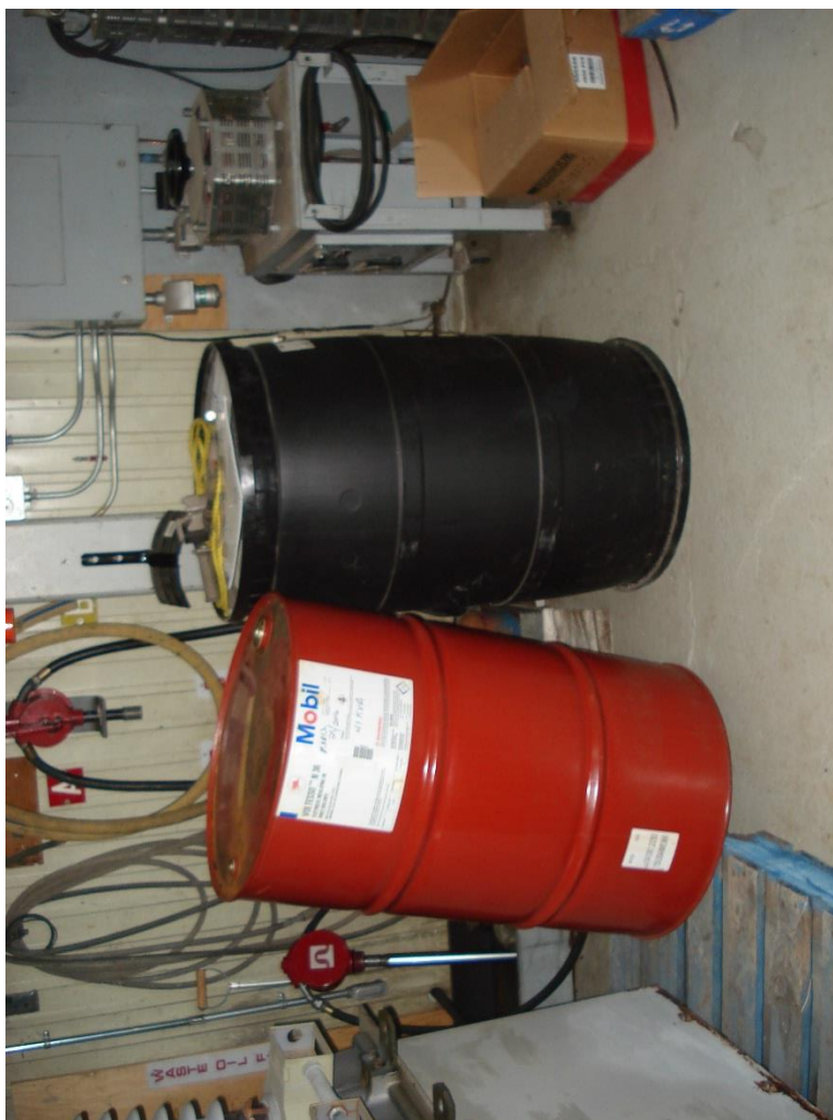
Photo 4 – Transformer Shop Oil Drums
