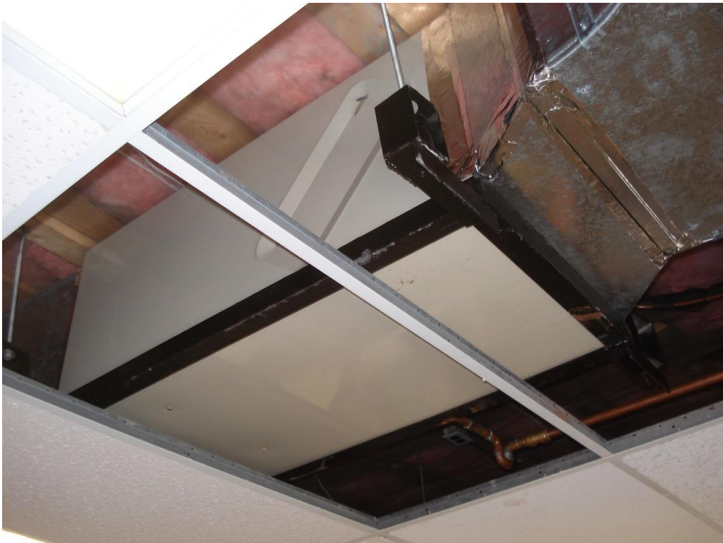
Photo 28 - Front Office Area Evaporator Unit
