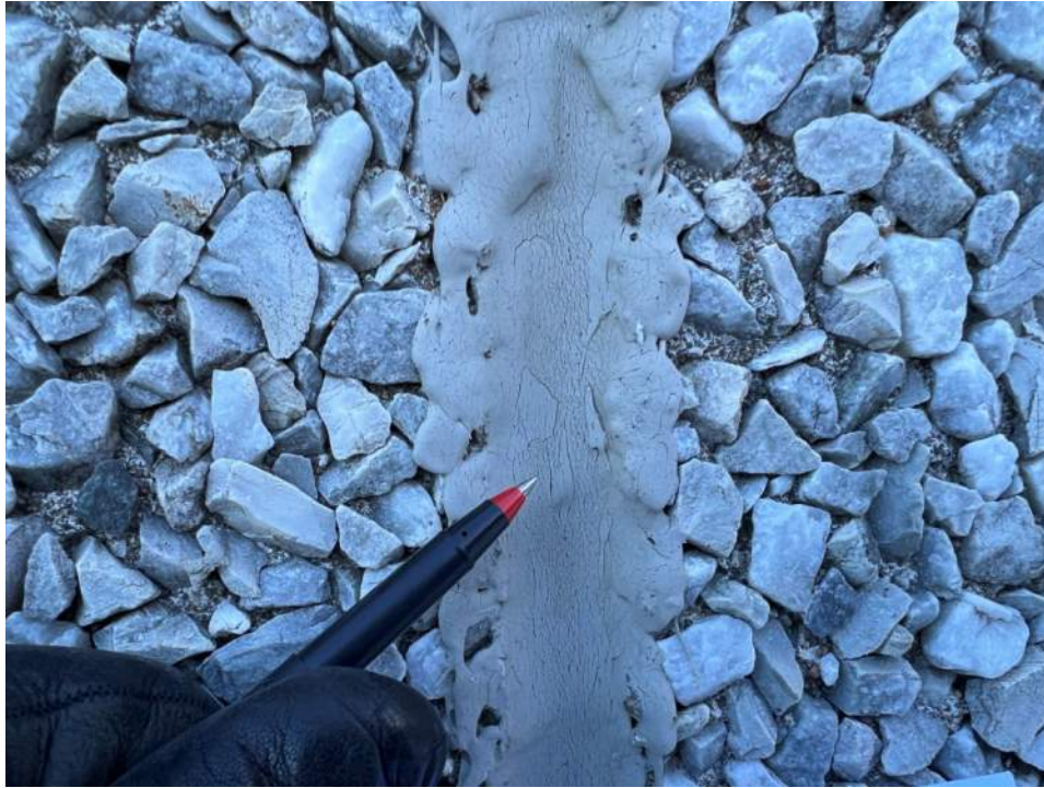
Photo No. 21: Typical view of localized precast panel joints crazing, and cohesive failures
