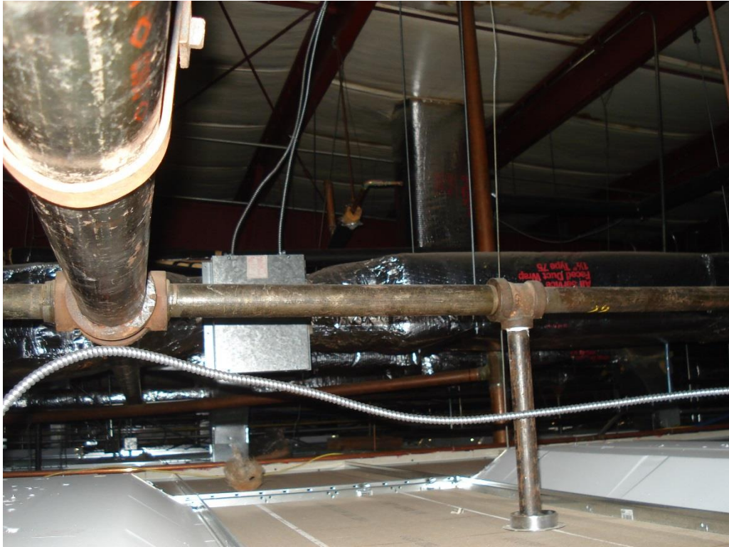
Photo 1 - Copper Vent Piping
