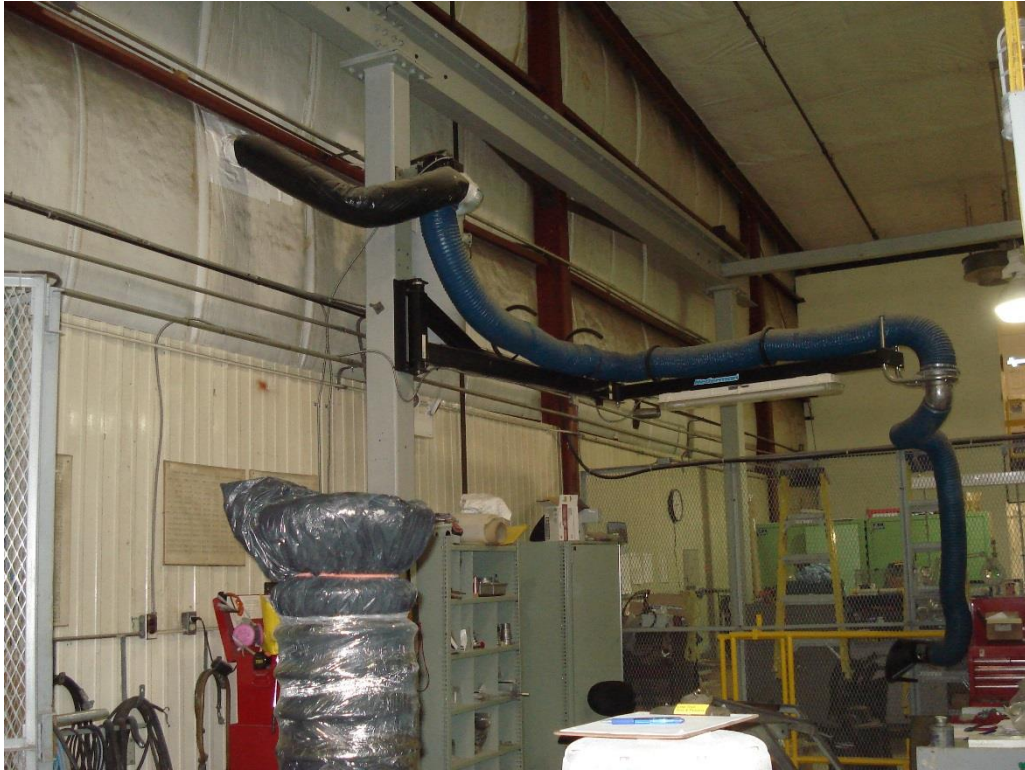
Photo 35 - Fume Extraction System
