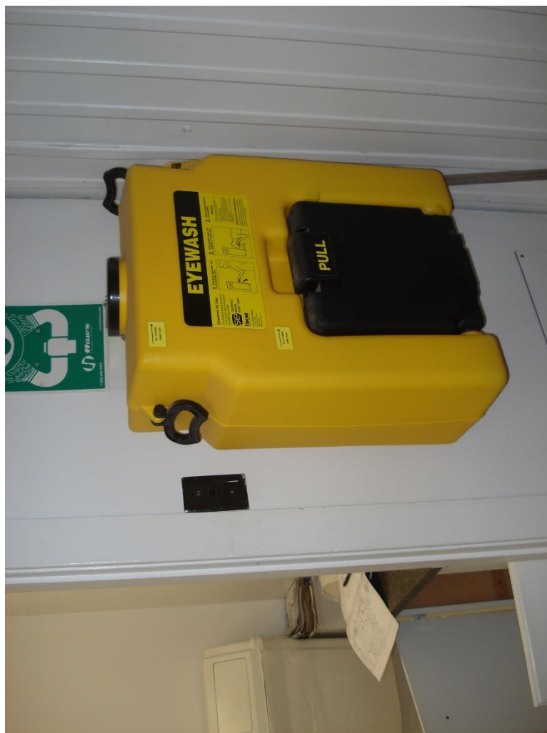
Photo 20 - Emergency Eyewash Station
