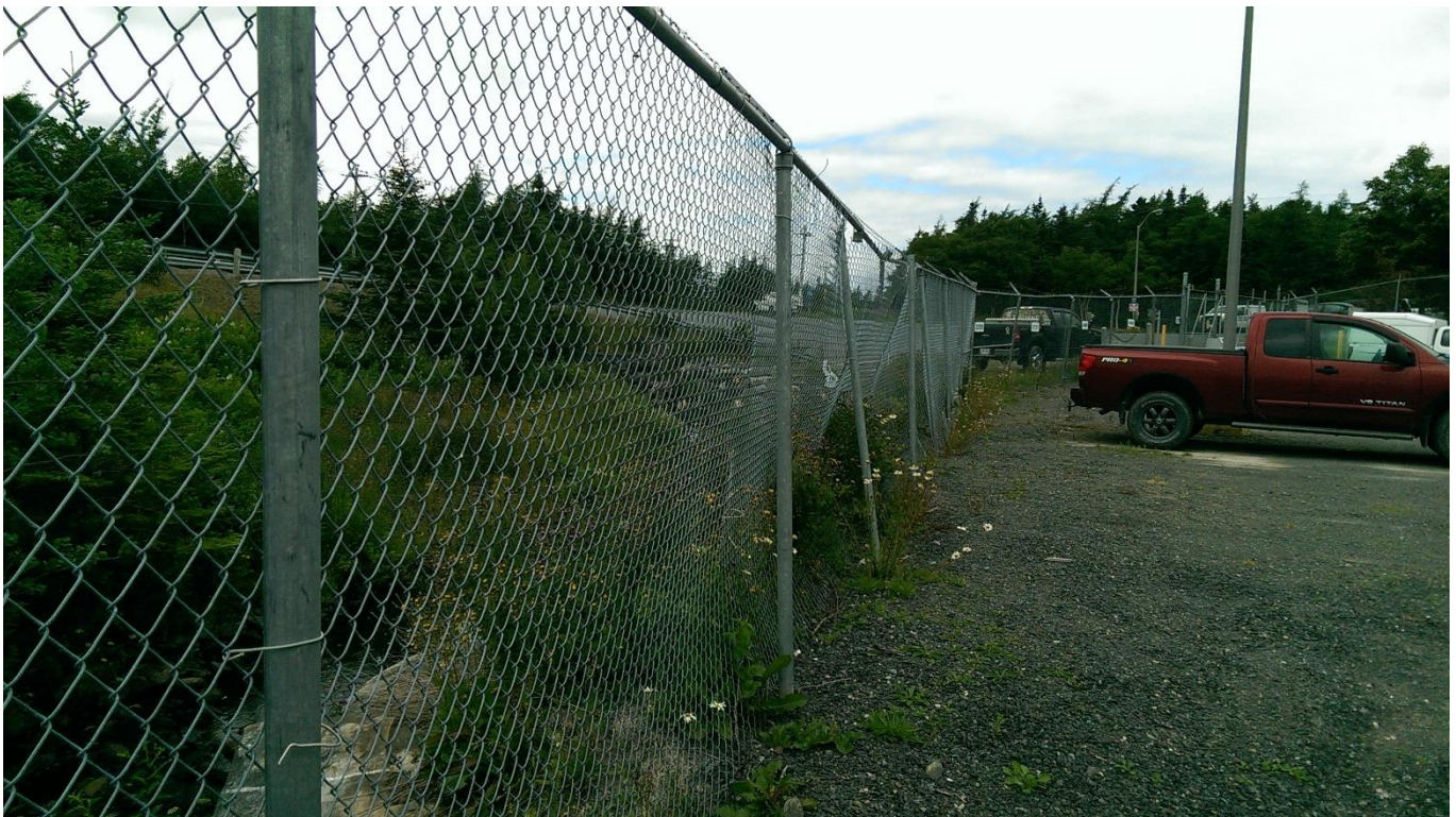
Photo 16 - Fence Leaning and Off From Bottom
