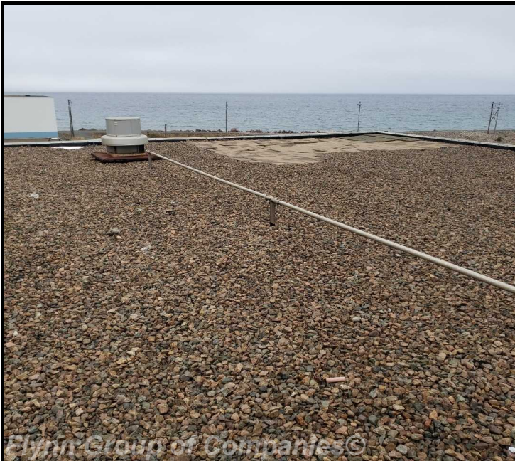
pump house #2: Overall clean
