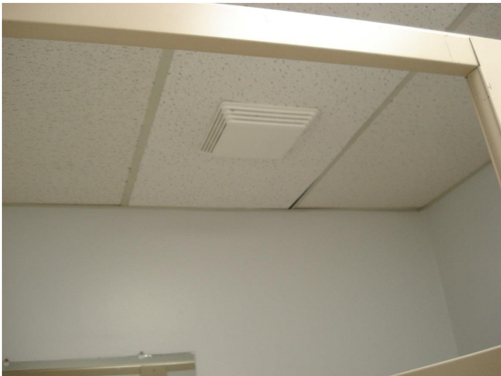
Photo 36 - Typical Washroom Exhaust Fan
