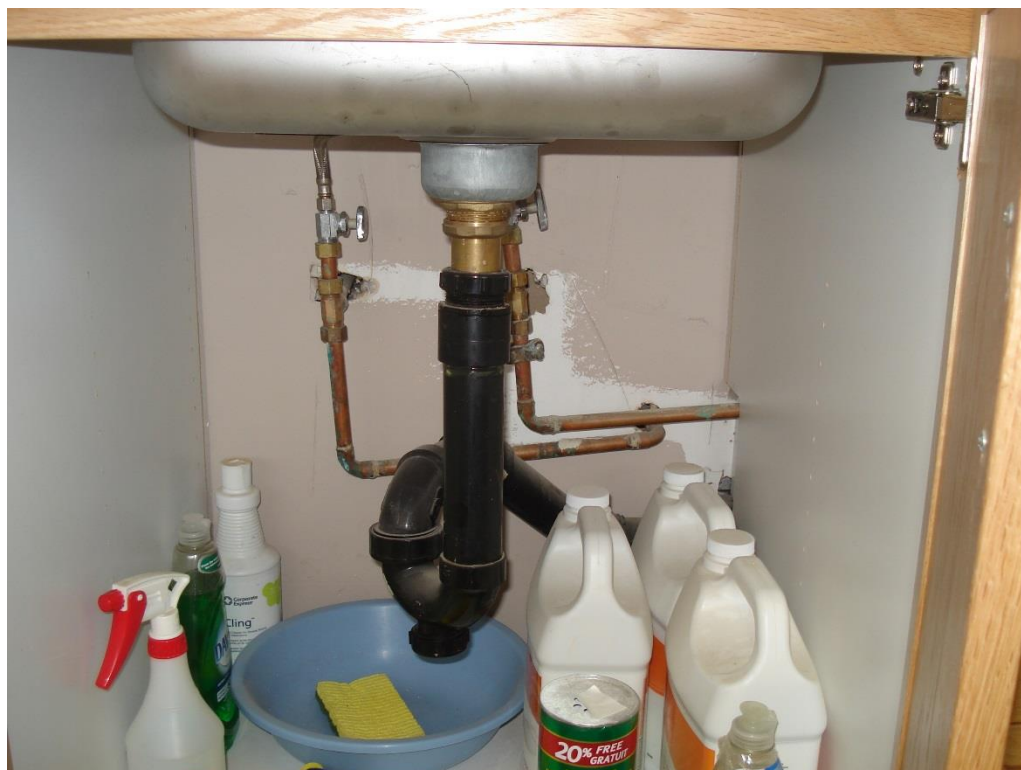
Photo 2 - ABS Drainage Piping
