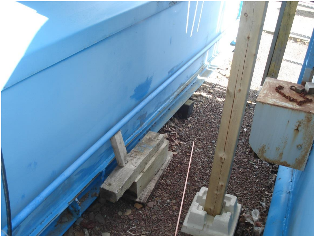
Photo 16 - Tank Piping Not Properly Supported
