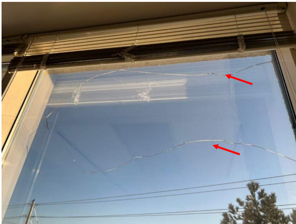
Photo No. 6: Typical view of cracked and showing an annealed breakage pattern windows (red arrows)
