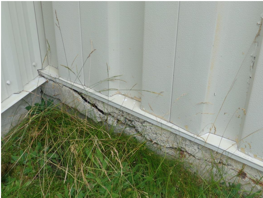
Photo 2 - Large Horizontal Cracks in Foundation
