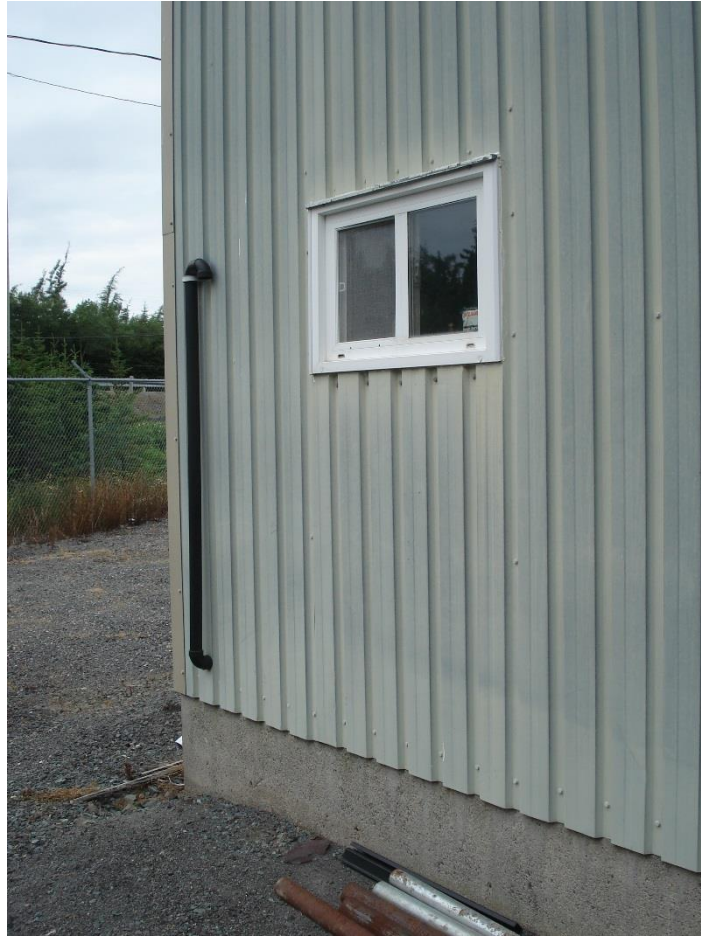
Photo 3 - Non Code Compliant Vent Piping
