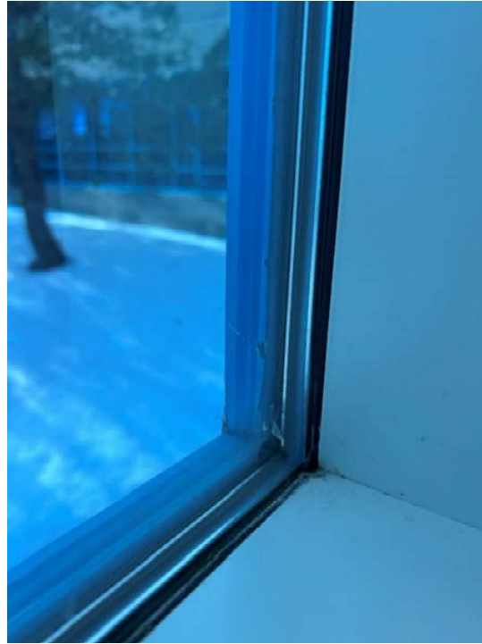
Photo No. 15: Typical view of interior glass-to-metal sealant is noted to be poor condition
