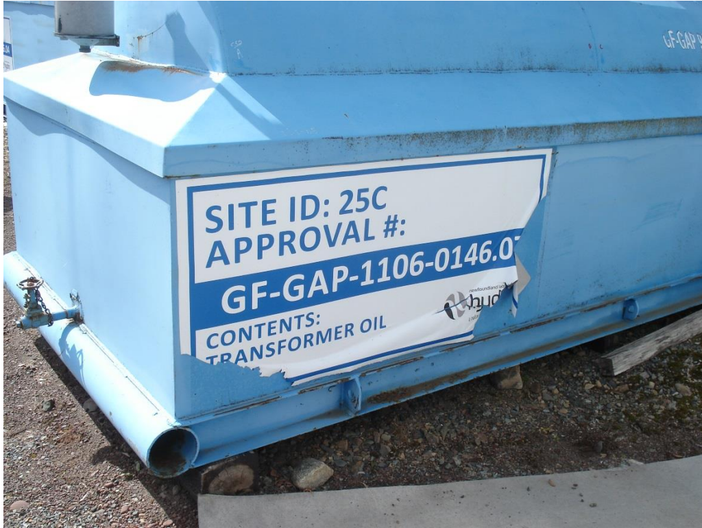
Photo 13 – 4,540 L Transformer Oil Tank
