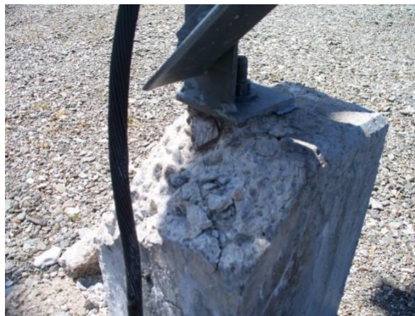
Figure 14: Structure B1T1 Bottom Brook Terminal Station
