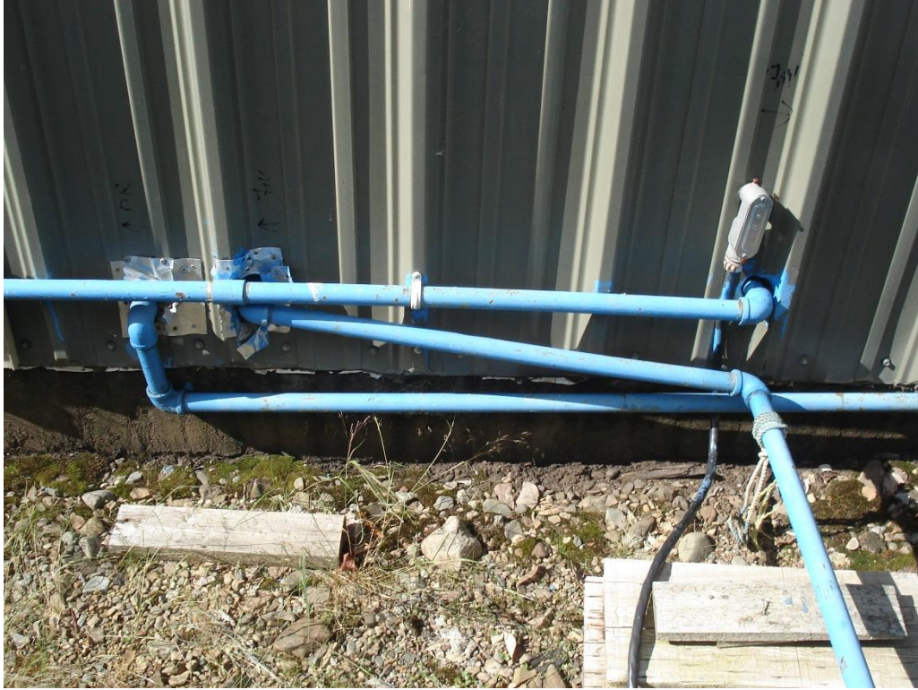
Photo 15 – Tank Piping Not Properly Supported
