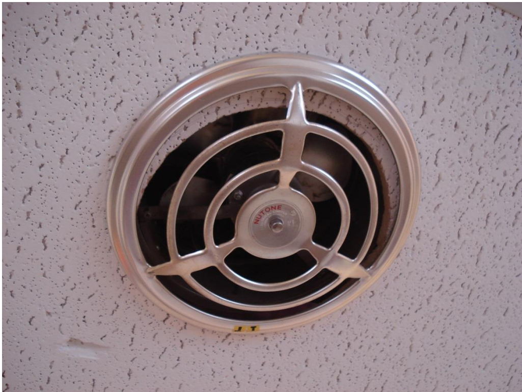
Photo 38 - Lunch Room Ceiling Exhaust Fan
