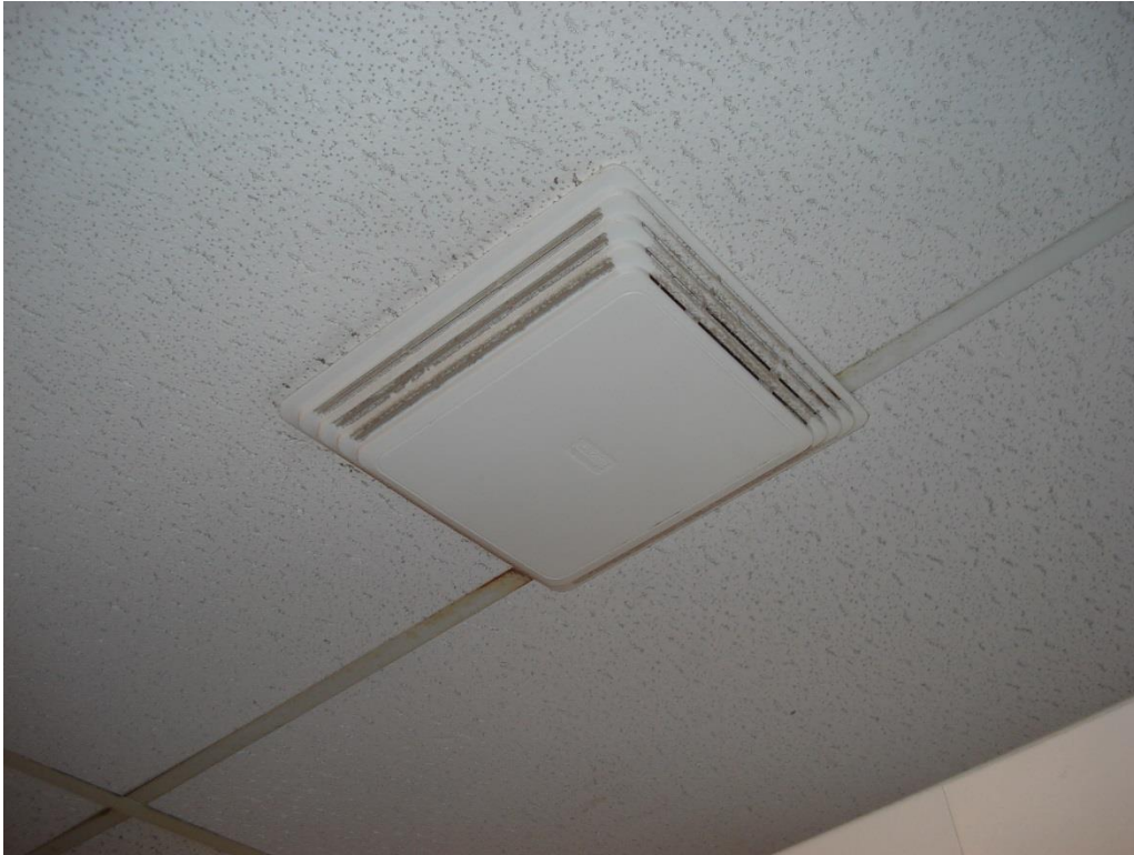
Photo 25 - Washroom Exhaust Fan
