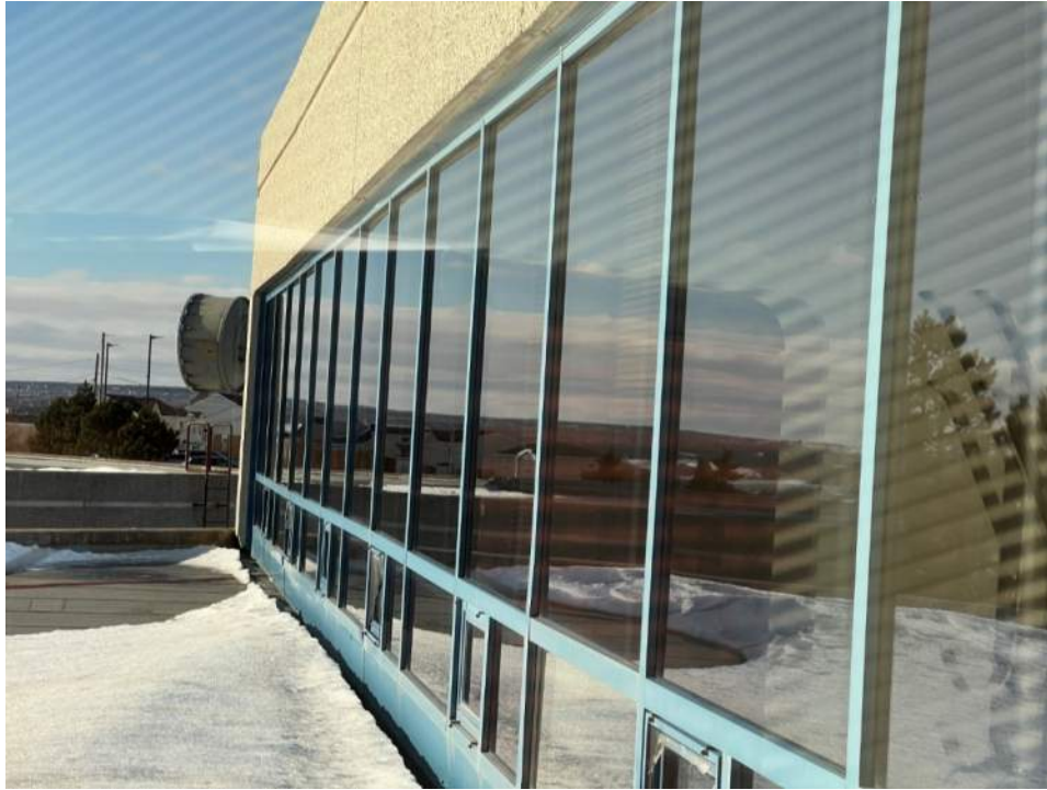
Photo No. 11: Typical view of curtain wall is in fair-to-poor condition overall with fading of the exterior caps
