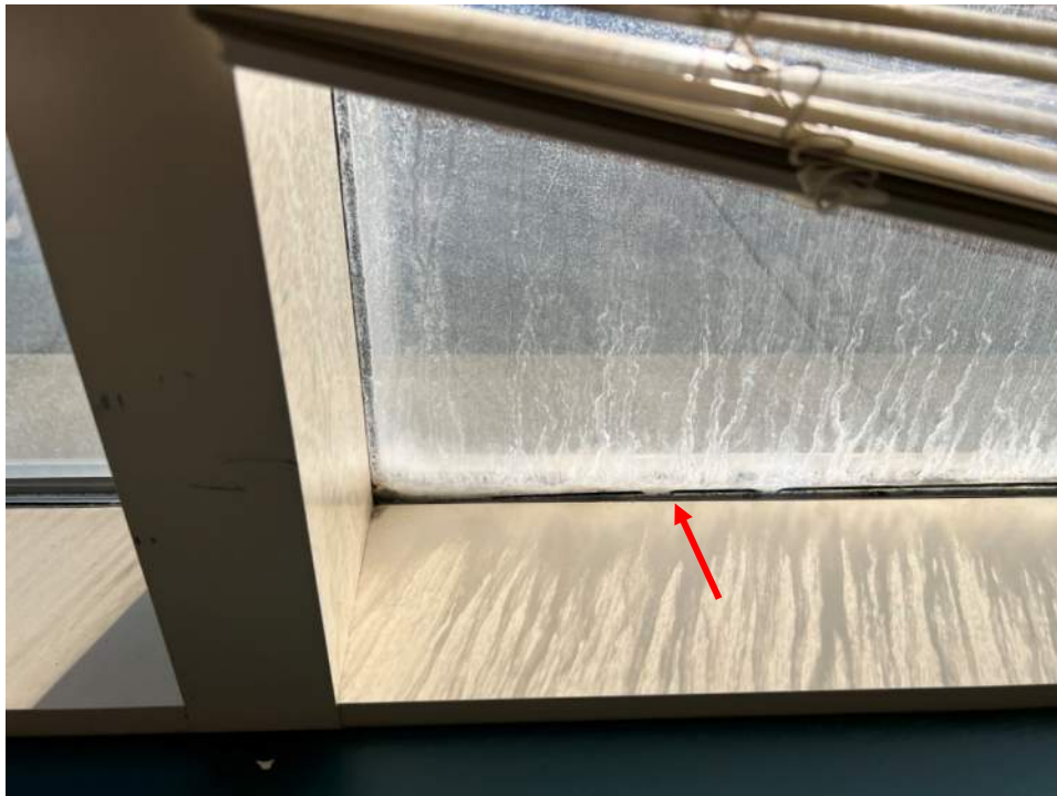
Photo No. 14: Typical view of interior glass-to-metal gasket is noted to be poor condition and failed IGU (red arrow)
