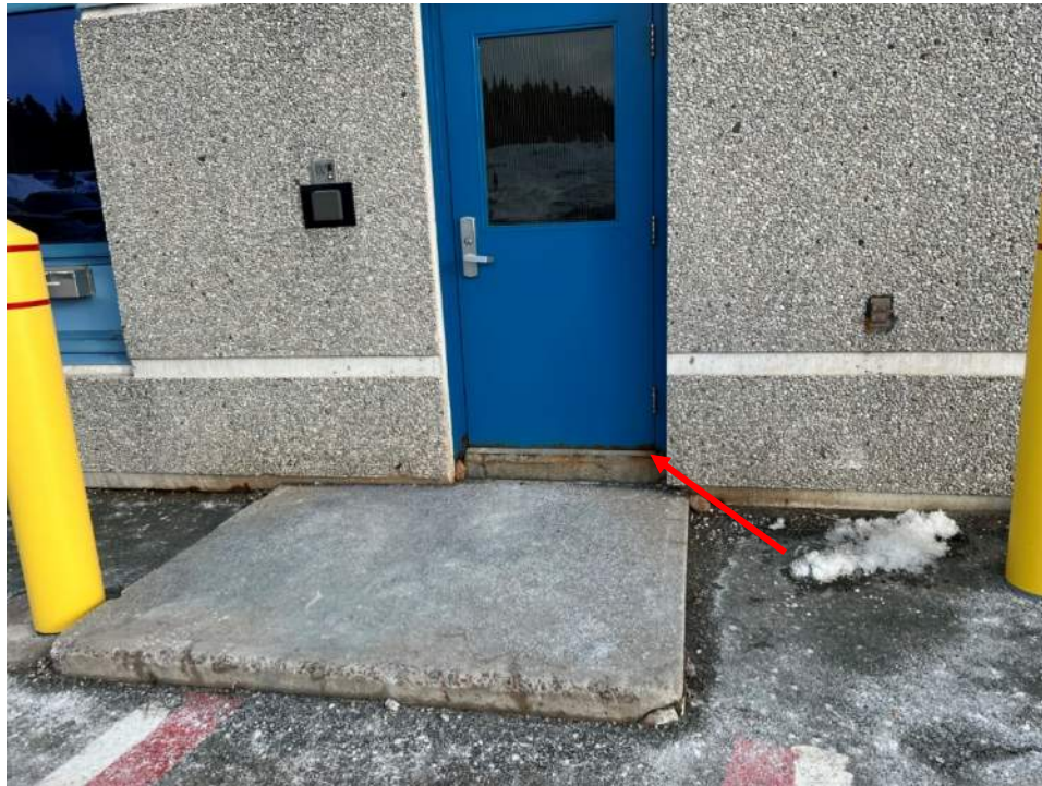
Photo No. 23: Typical view of anodizing is noted faded, and there is rust formation at the bottom of the doors (red arrow)
