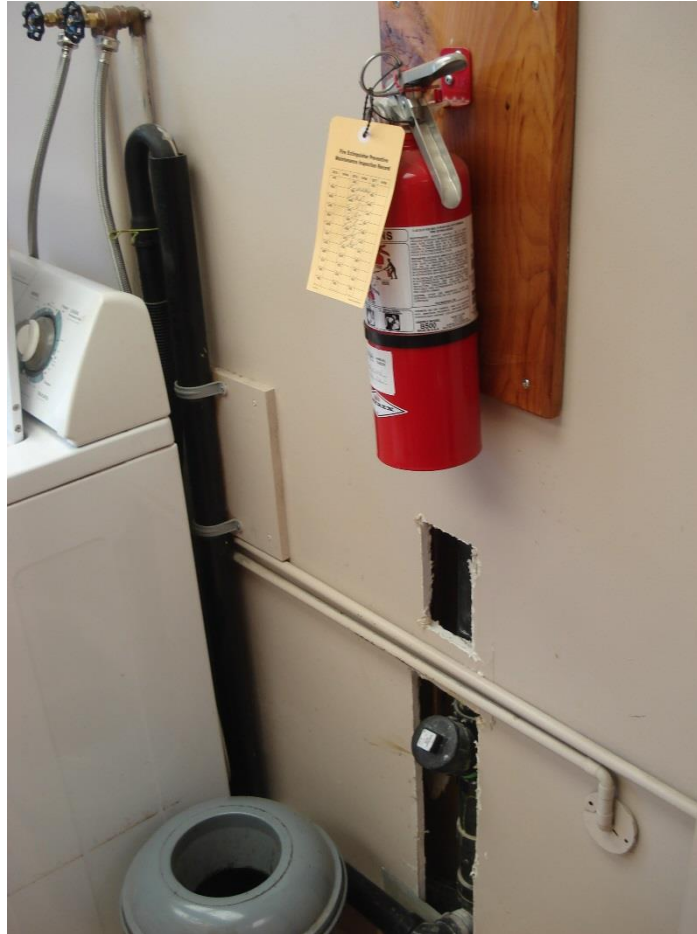
Photo 1 - ABS Drainage and Vent Piping
