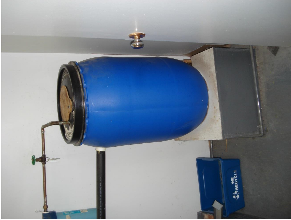
Photo 12 - Water Barrel on Mezzanine Level
