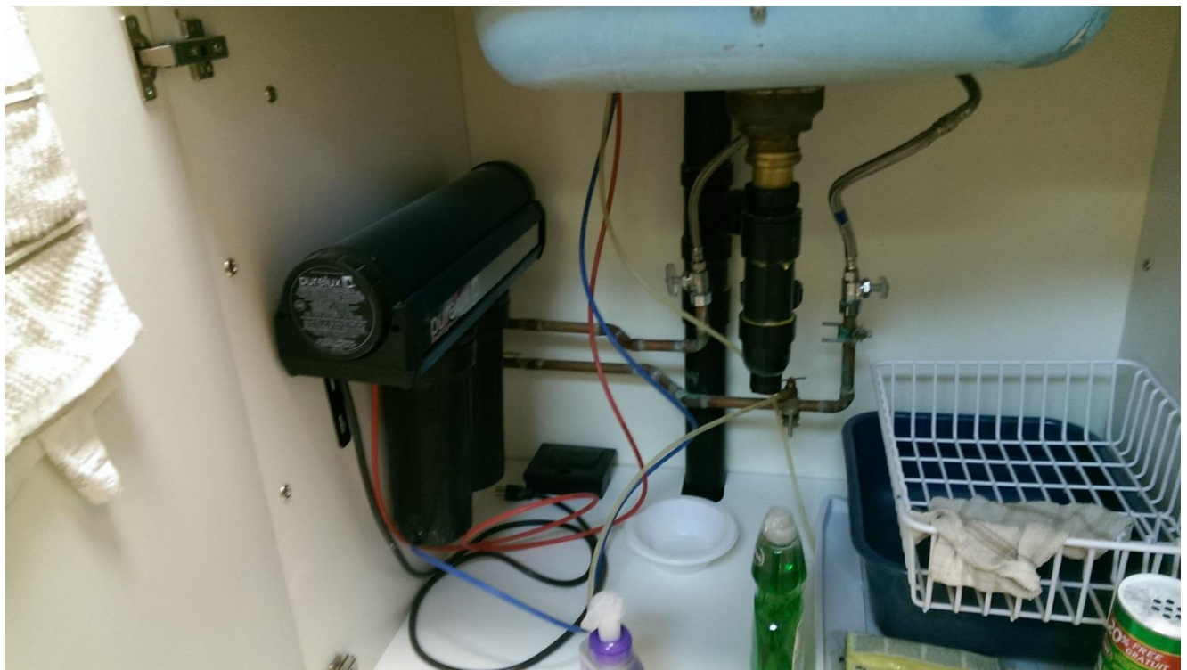
Photo 12 - Lunch Room Sink Water Filtration System
