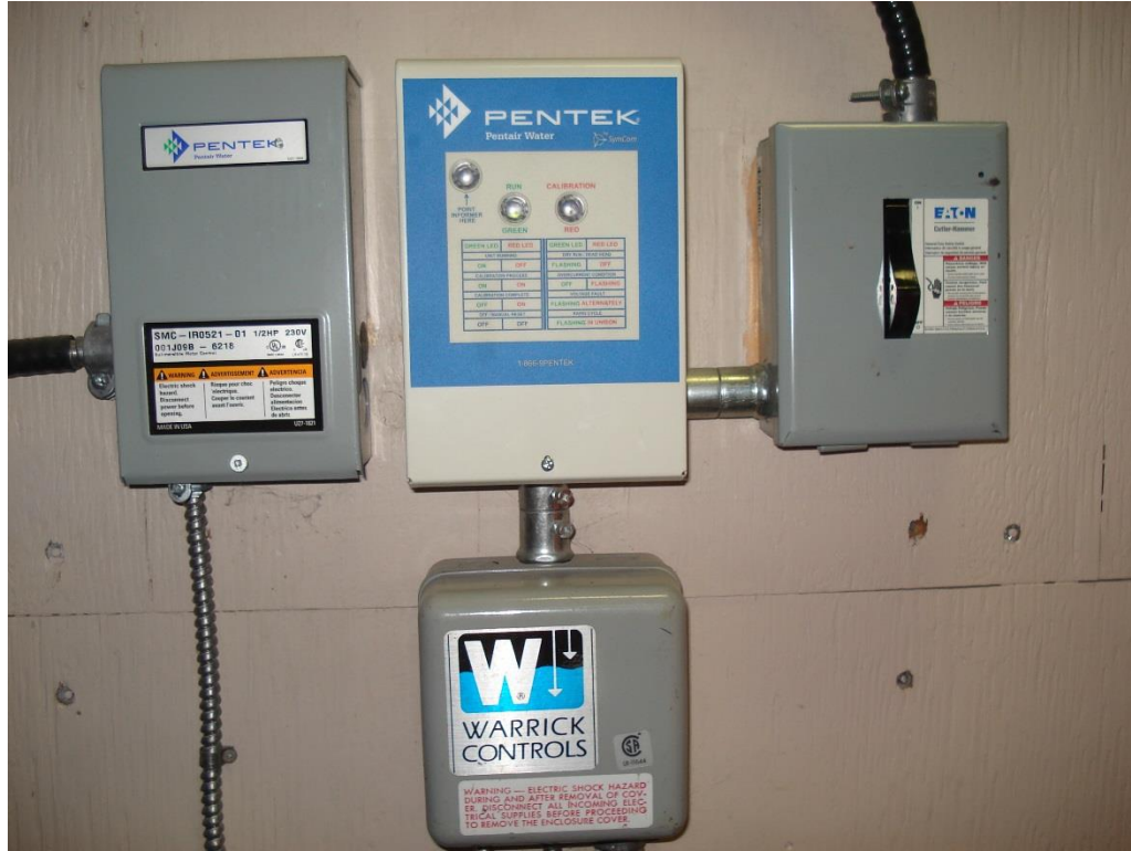
Photo 9 - Well Pump Controls
