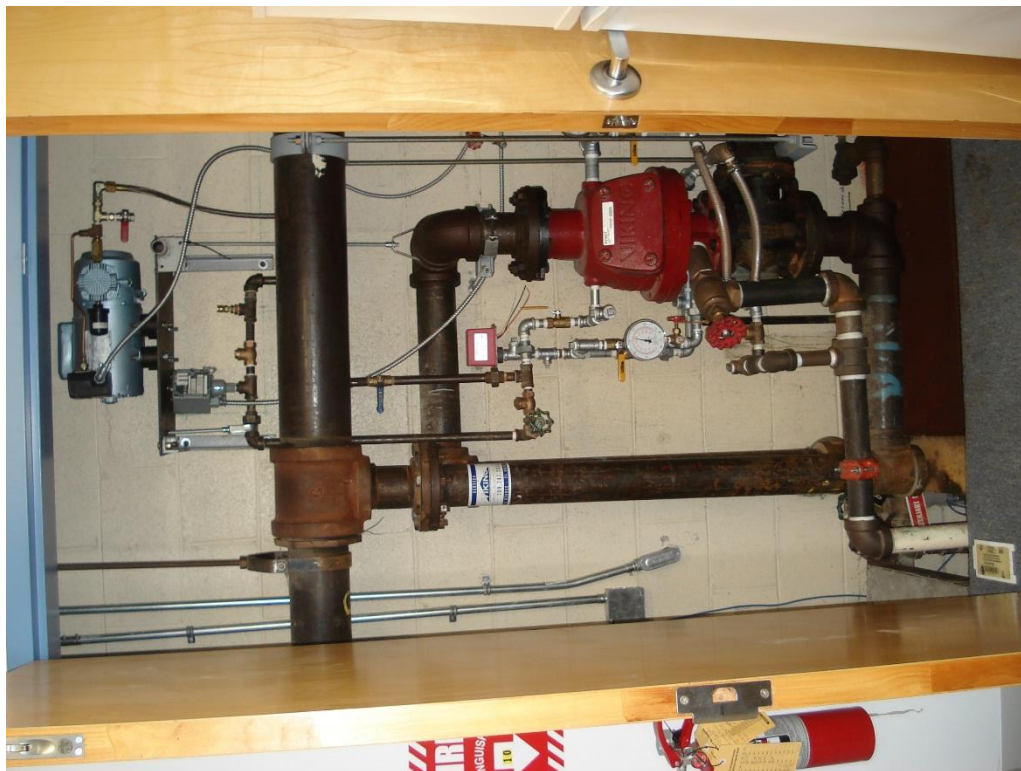
Photo 46 - Dry Sprinkler System Valve
