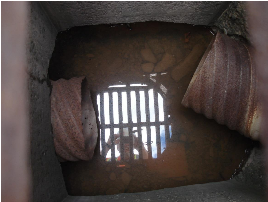
Photo 12 - Catch Basin Chamber Undermined
