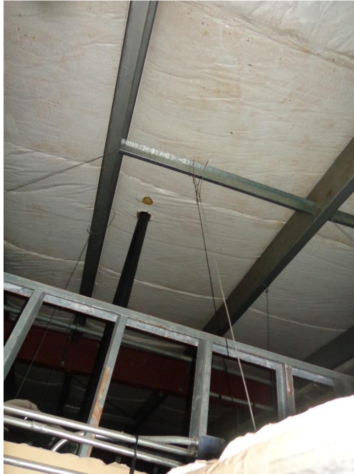
Photo 3 - ABS Vent Piping
