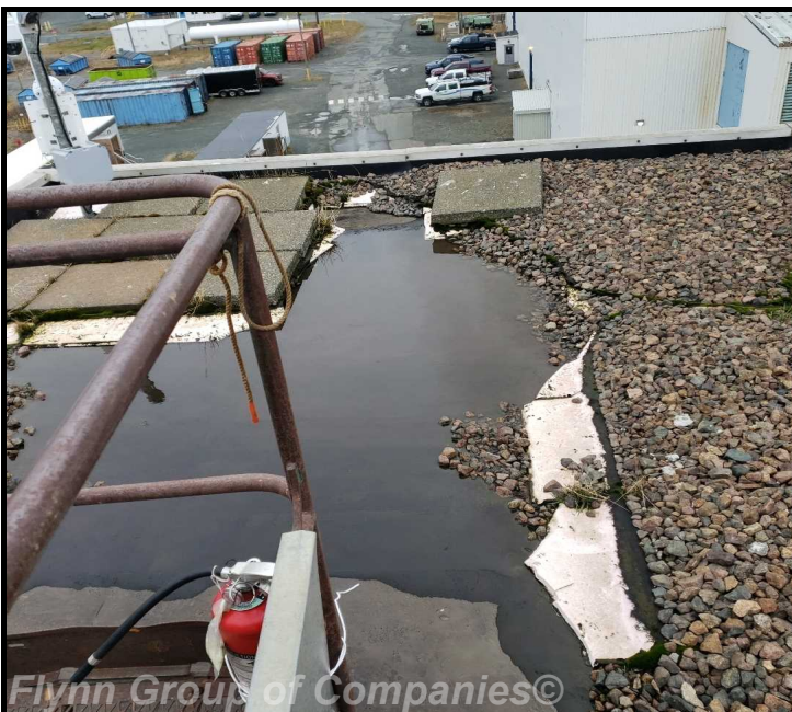
pump house #2: View of wind blown area to be addressed
