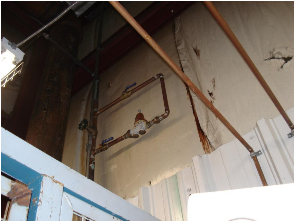
Photo 6 - Domestic Water Entrance
