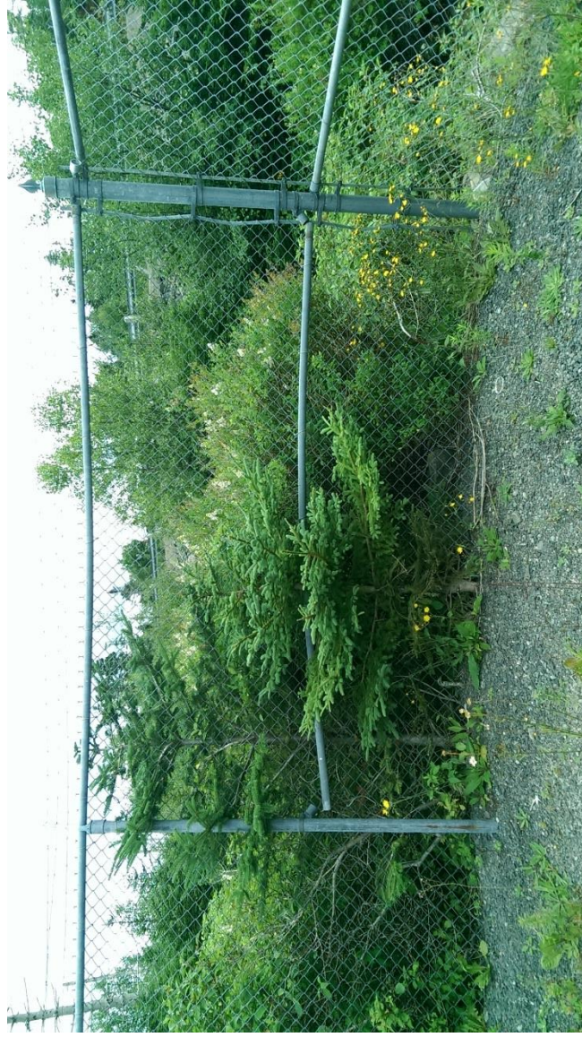
Photo 14 - Braces Bent and Off
