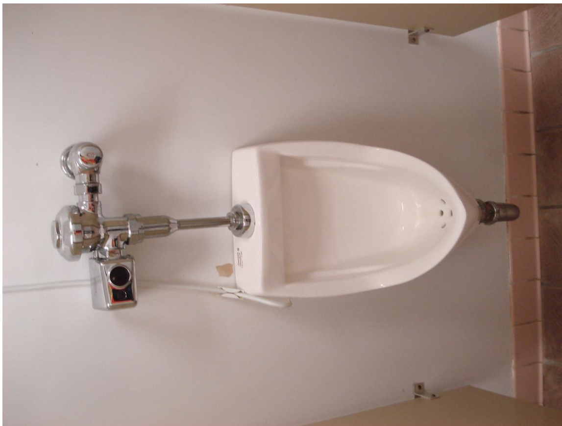
Photo 14 - Urinal with Electronic Flush Valve
