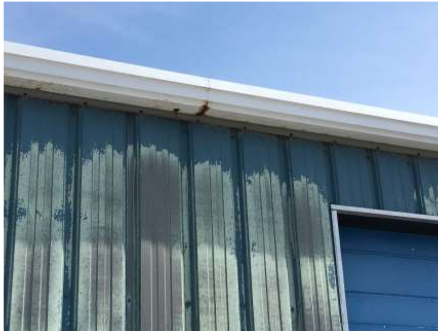
Corroded soffit and paint peeling from cladding.
