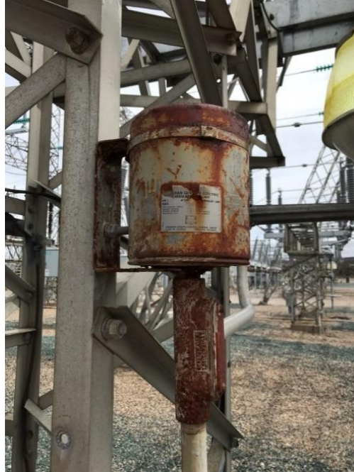
Figure 12: Corroded Ballast Requiring Replacement
