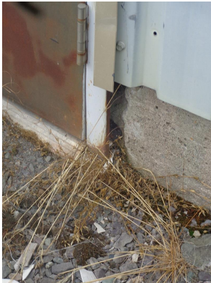
Photo 2 - Concrete Spall on Foundation Wall
