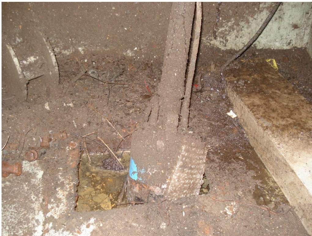
Photo 4 - Service Pit Sump Pump
