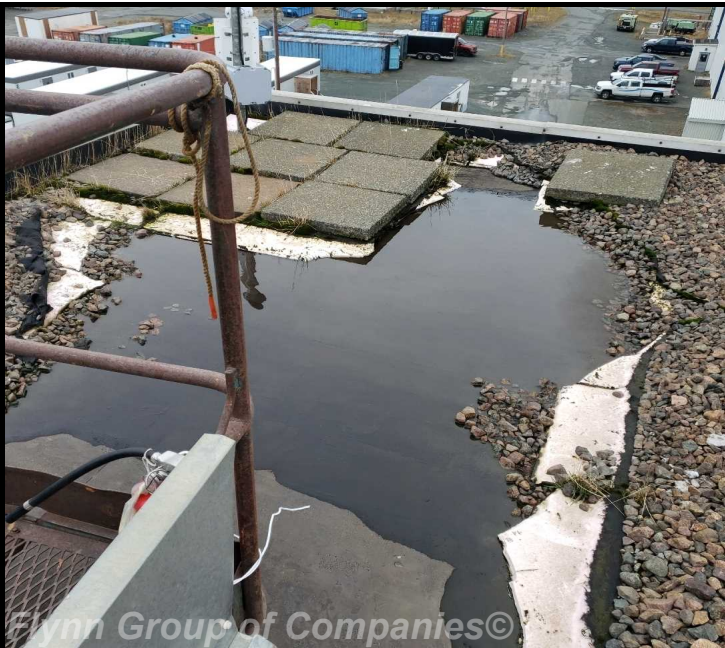
pump house #2: Area of wind damage
