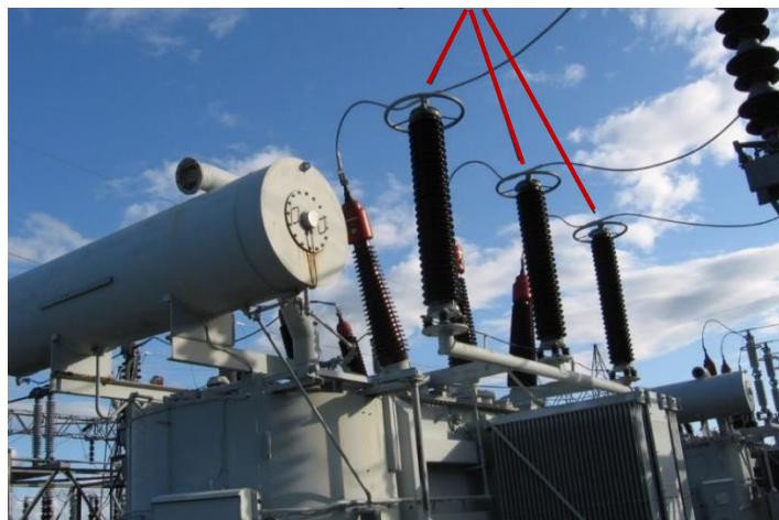
Figure 5: Western Avalon Terminal Station Transformer T3 230 kV Surge Arresters
