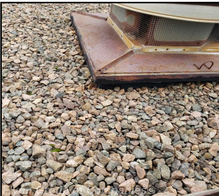
pump house #2: Penetration flashings
