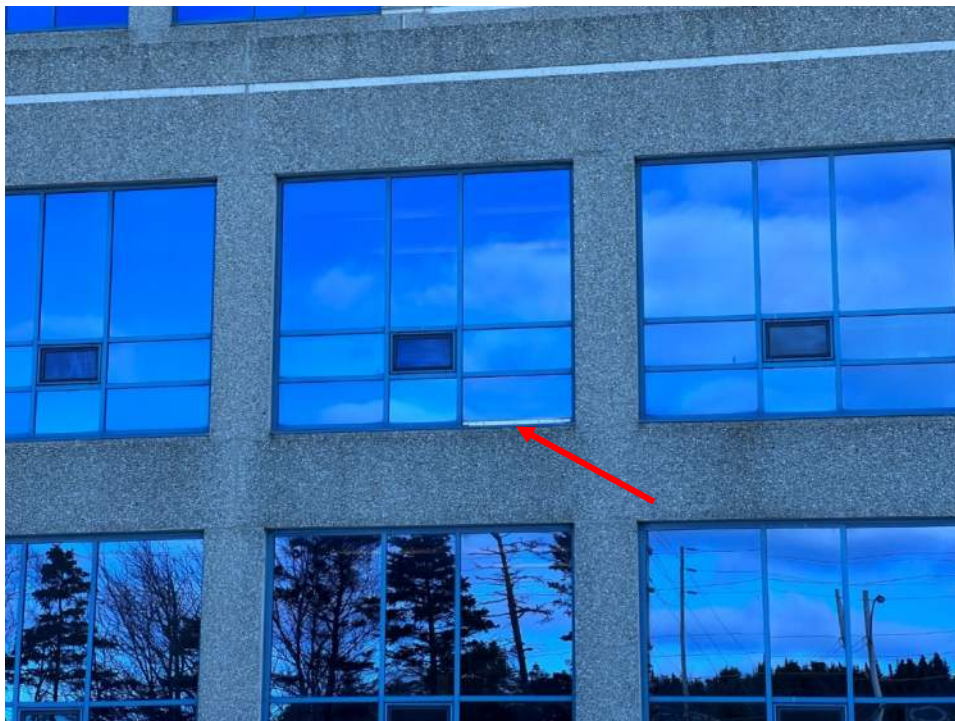
Photo No. 28: Typical view of punched windows in fair to poor condition with a missing snap cap (red arrow)
