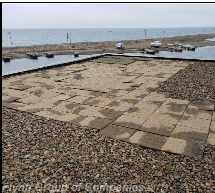
pump house #2: View of area of paving stones at corner of parapet
