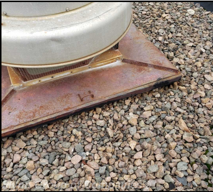
pump house #2: Areas of open seams to be caulked on fan curbs and parapet metal
