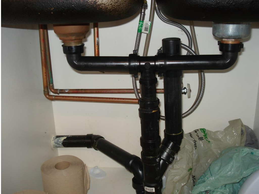
Photo 3 - Air Admittance Valve Mounted Incorrectly
