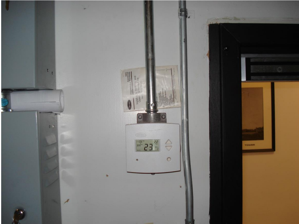
Photo 43 - Typical Split AC System Thermostat
