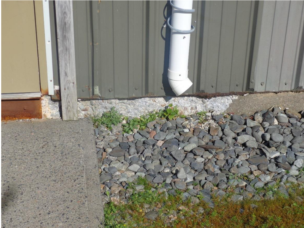
Photo 3 - Scaled Concrete on Foundation Wall
