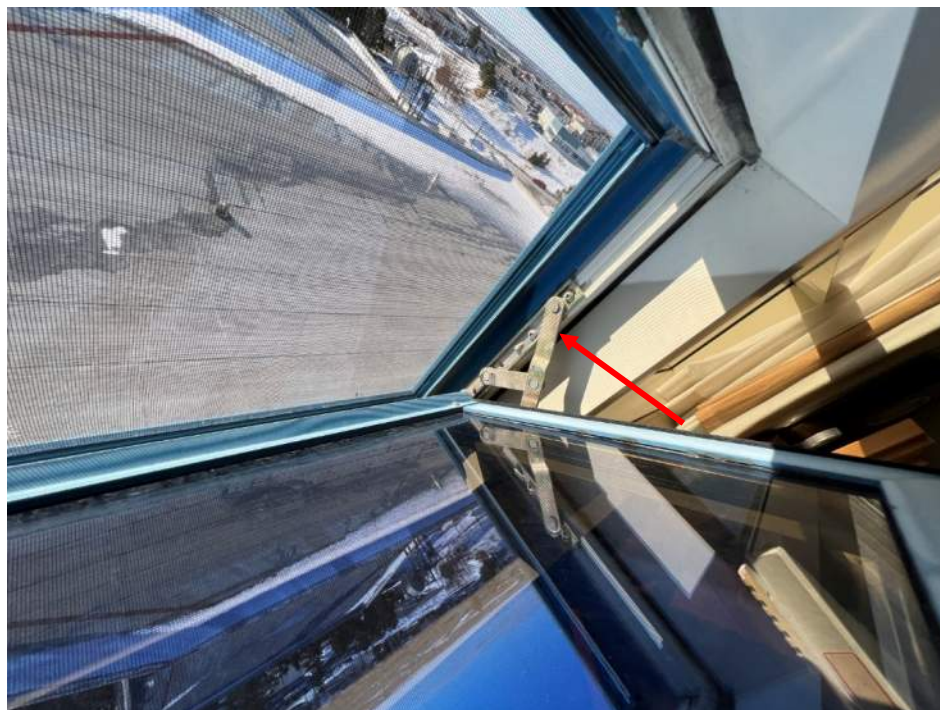
Photo No. 18: Typical view of rusted roto gear (red arrow)
