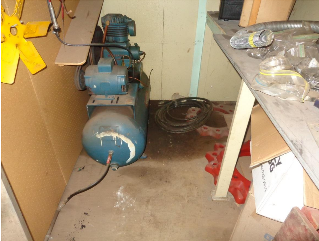
Photo 5 - Moisture or Staining by Equipment
