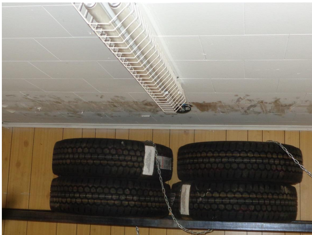
Photo 2 - Marks Made by Tires on Ceiling
